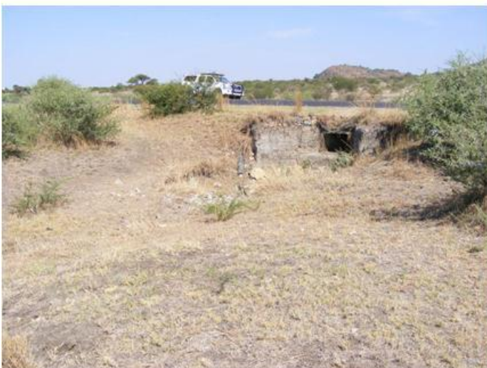
Figure 30: Tierkop Spruit - The culvert constructed to allow storm water from the drainage line to pass through.
