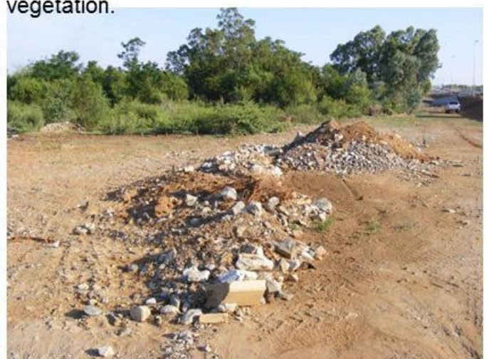
Figure 17: Dorp's River - Development on the outskirts of the riparian woodland - road building.
