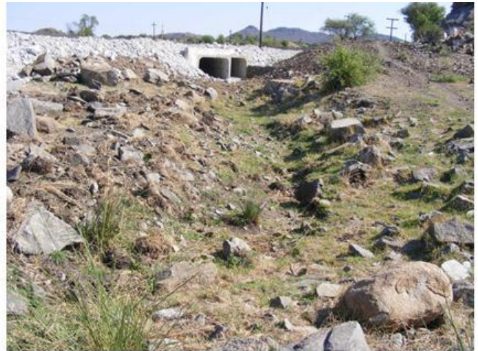
Figure 27: Kanana drainage - The culvert constructed to allow storm water from the drainage line to pass through.
