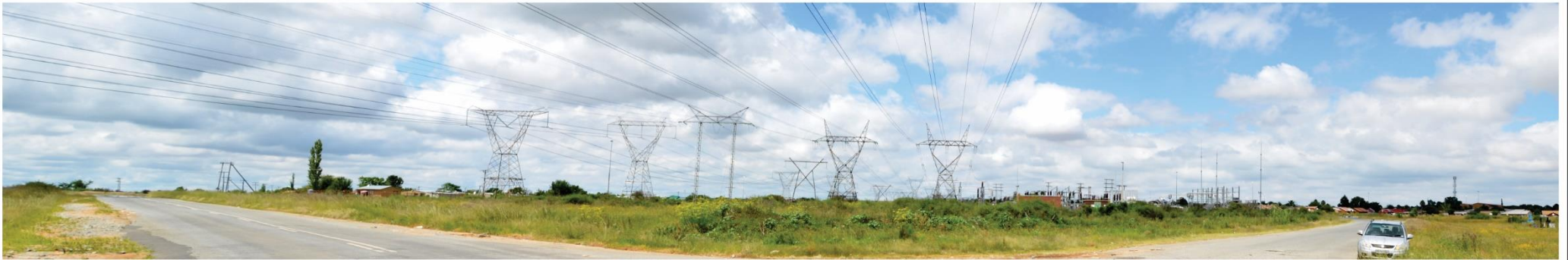
CL 237 looking northwest towards the existing substation at the entrance to the township of Meloding
