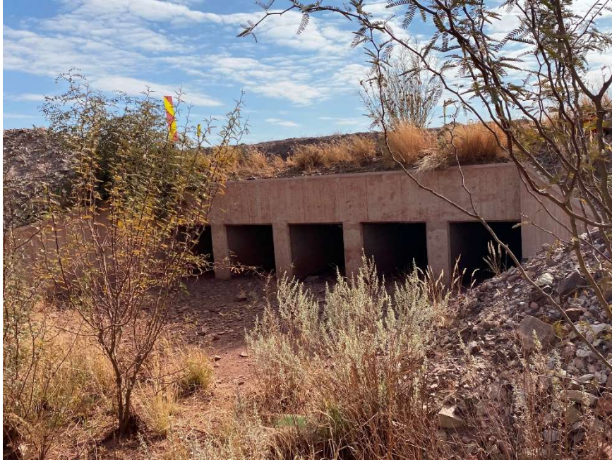
Figure 28 : Haul Road, five-barrel culvert near Kapstevl
