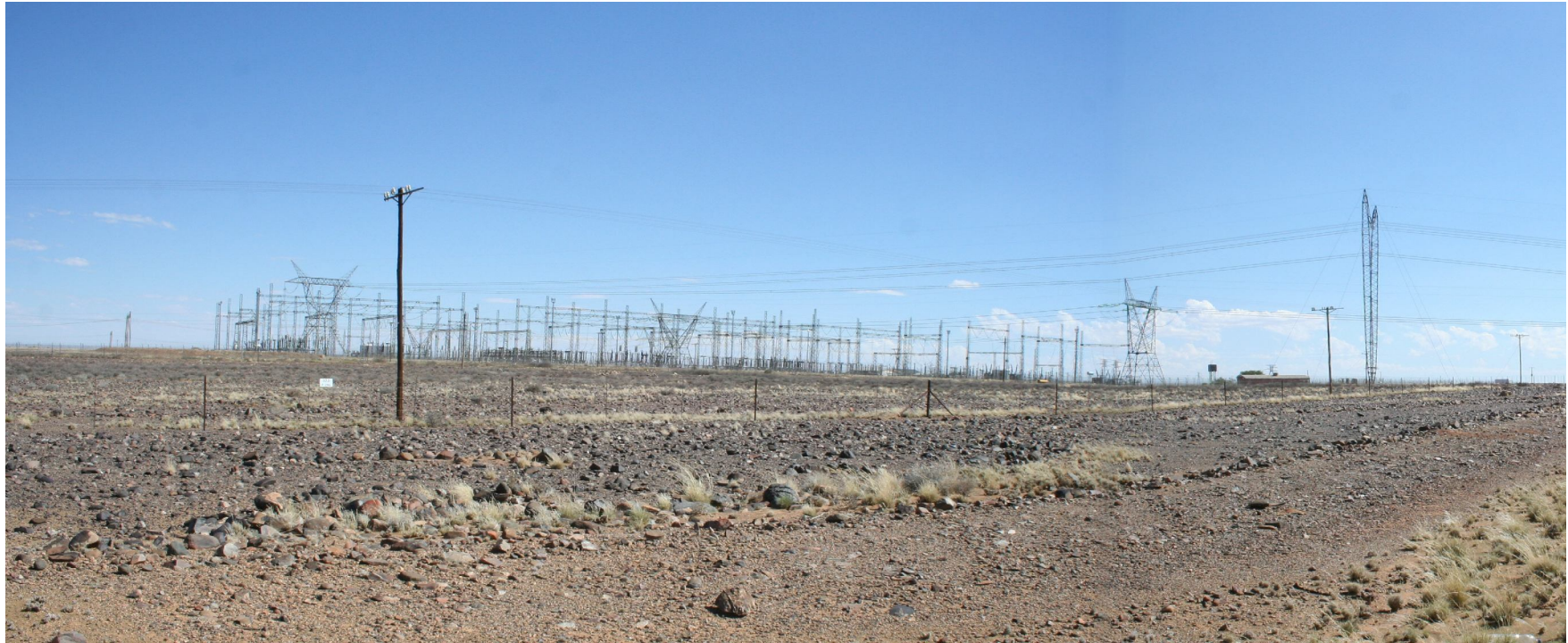
Aries substation as seen from Kenhardt / Pofadder road
