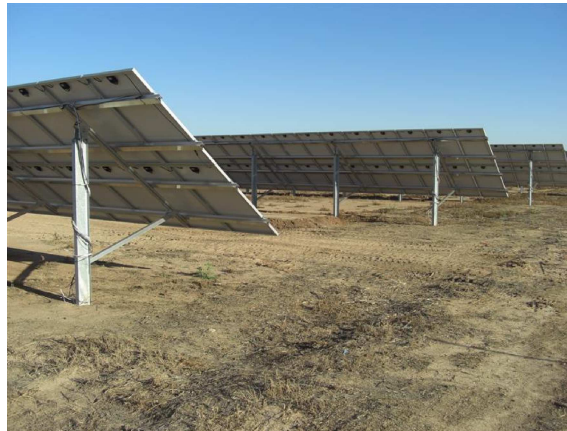
Back view of solar panels
