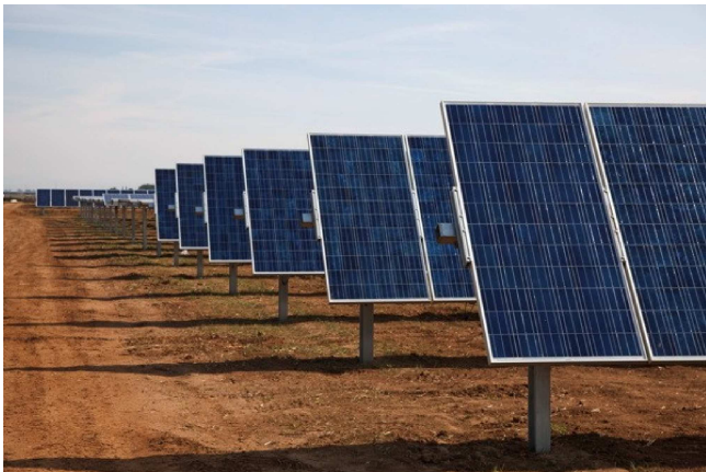
Front view of solar panels
