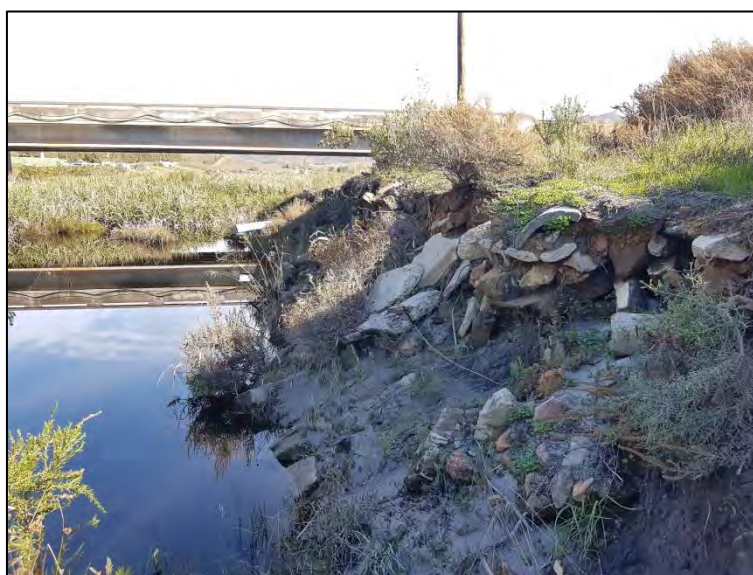
Figure 1.8.1 Proposed unstable bank to be stabilised with sloping and installation of groynes
