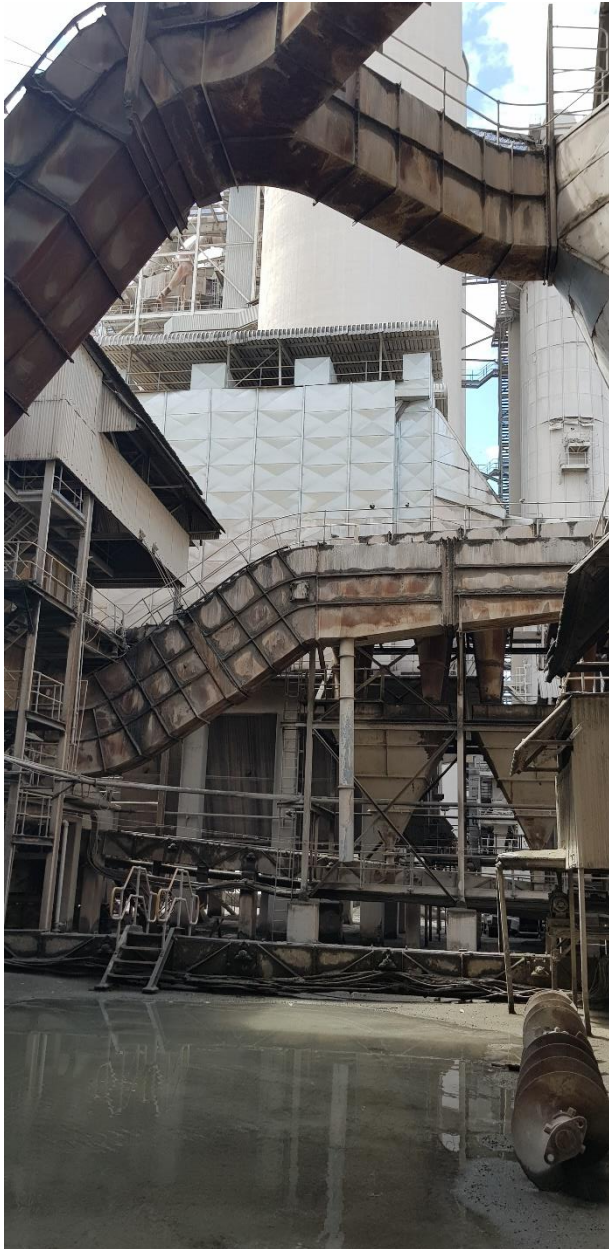
Figure 3: Example of Associated Infrastructure (Electrofilter)
