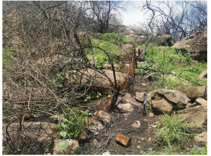
Dilapidated fence along the massive rock outcrop
