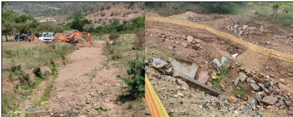
Figure 29: Excavation and earth works within the river channel and drainage lines respectively (November 2019)
