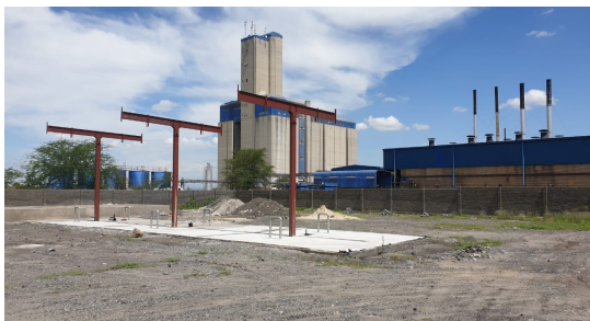
16. View of the activity unlawfully commenced with – above and to the right. Commencement of construction of pillars of forecourt
