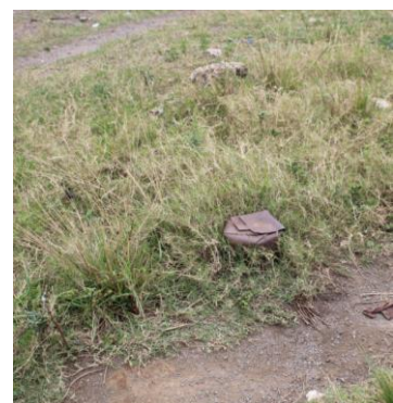
Figure 9: Capped manhole without additional protection
