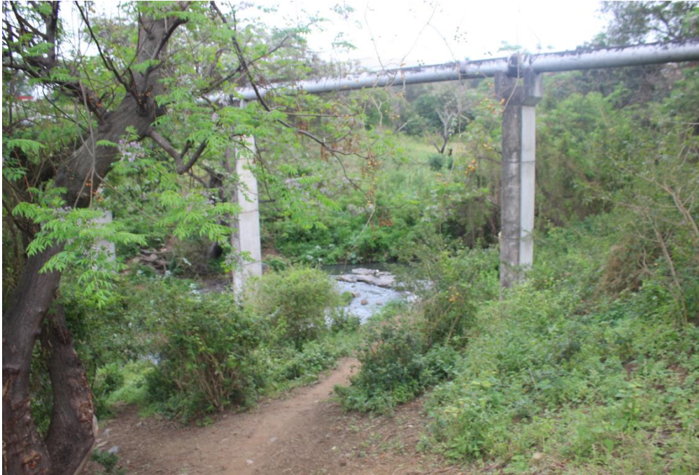
Figure 10: Sewerline traversing the site and crossing a tributary of the Mbozamo River
