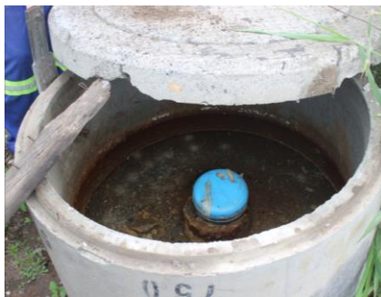
Figure 8: Monitoring borehole protected by a manhole
