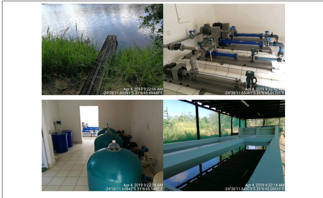
Figure 2: Images of water abstraction pump and purification system
