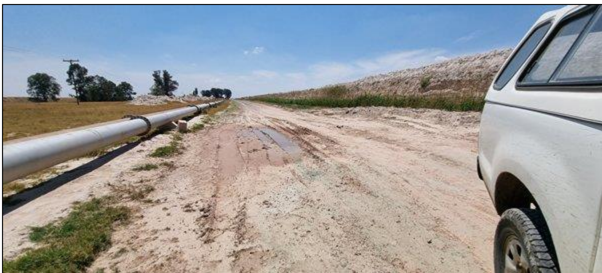
Figure 7-3 Examples of artificial wetlands formed due to leaking pipes and sewage infrastructure
