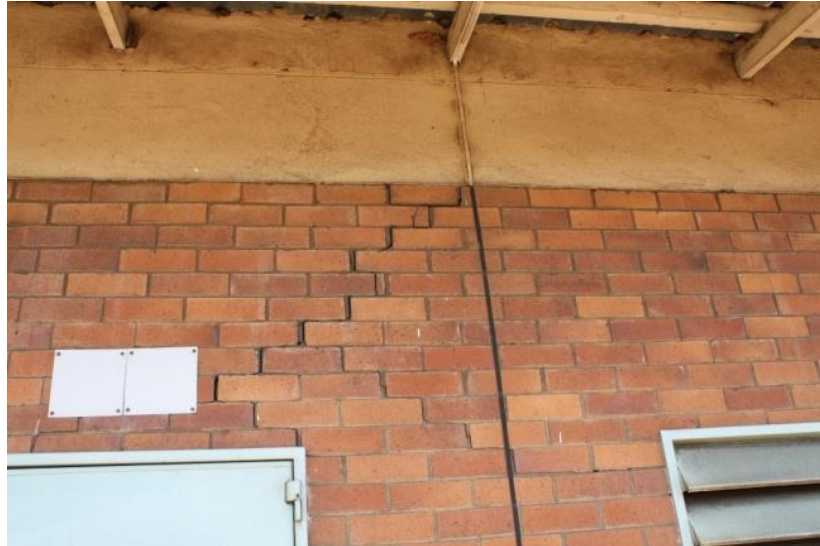
Figure 15: Example of blast induced damage.
