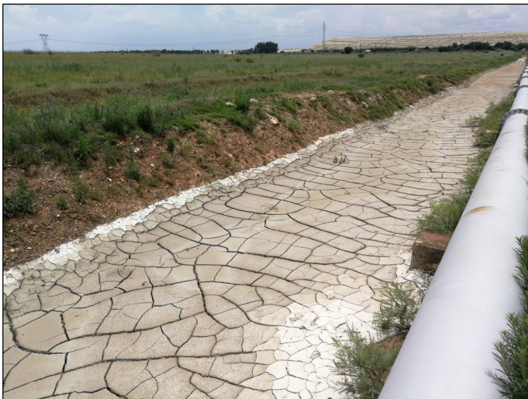
Figure 6-1 Photograph showing evidence that the existing pipeline has been leaking into the surrounding environment
