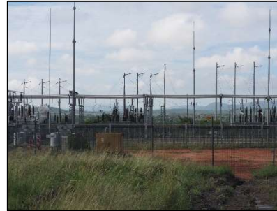
Figure 9: Electrical substation to the north-east of the study area.
