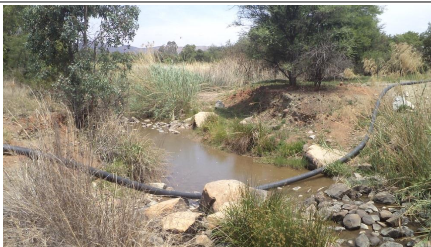
Figure 5: Pipe transferring water from west pit to HERNIC Open pit over the Sterkstroom River
