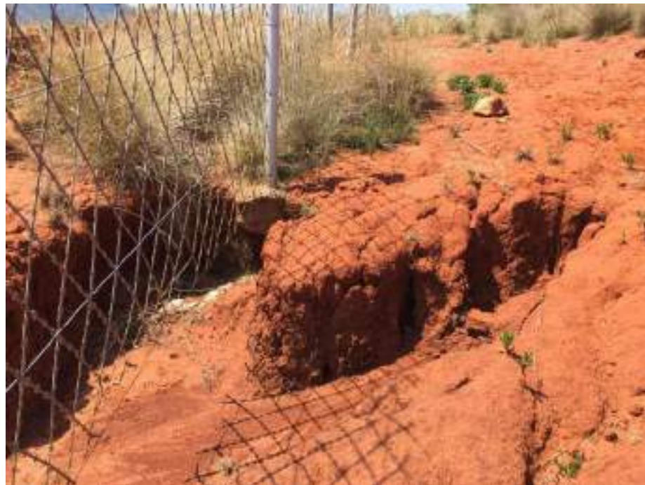
Figure 8: Active erosion of the residual soil as shown by erosion of the western boundary fence post foundation.
