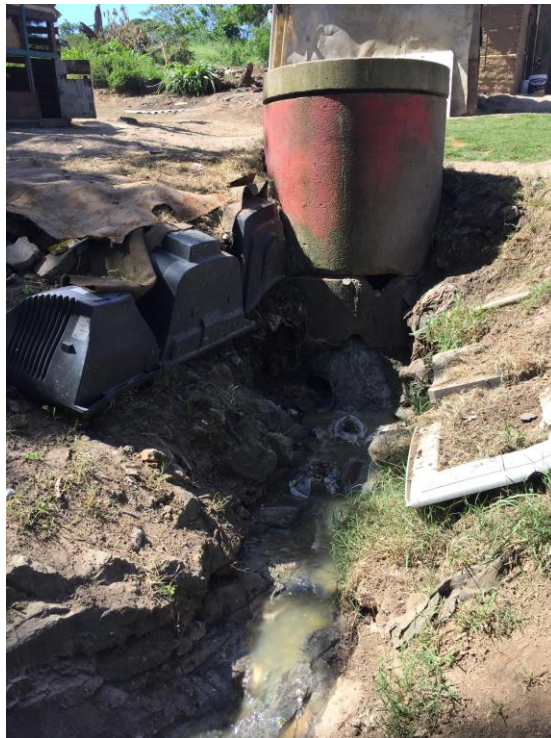
Figure 19: A burst sewage pipe leaking straight into a stream.
