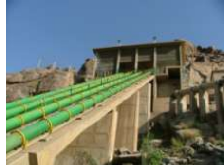
Henkries River Pump Station
