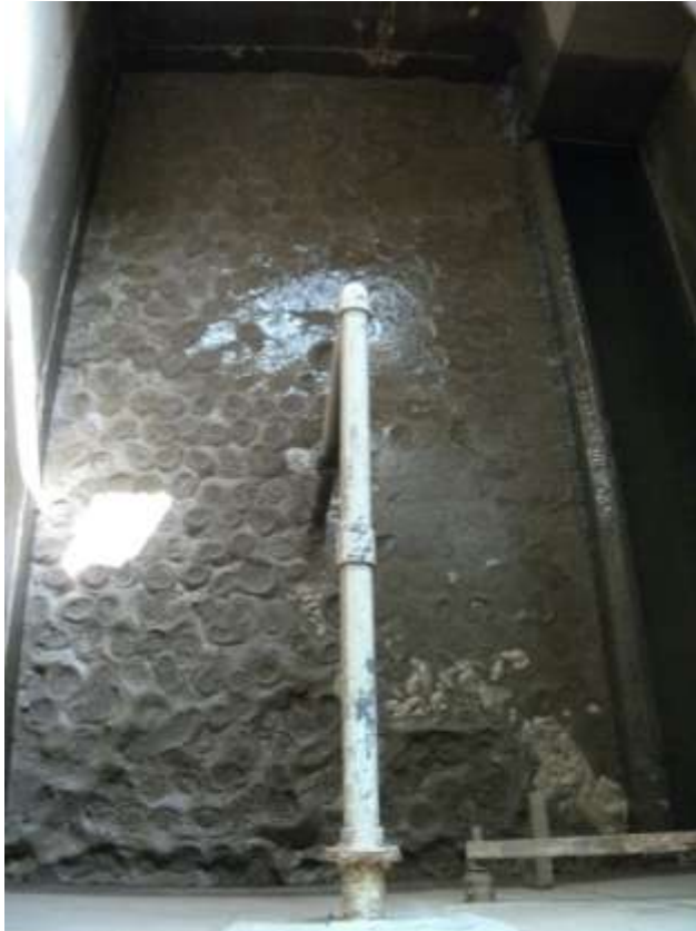
Typical filter surface at Henkries WTP
