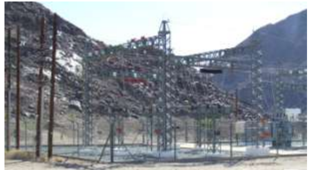
Henkriesmond Electrical Substation
