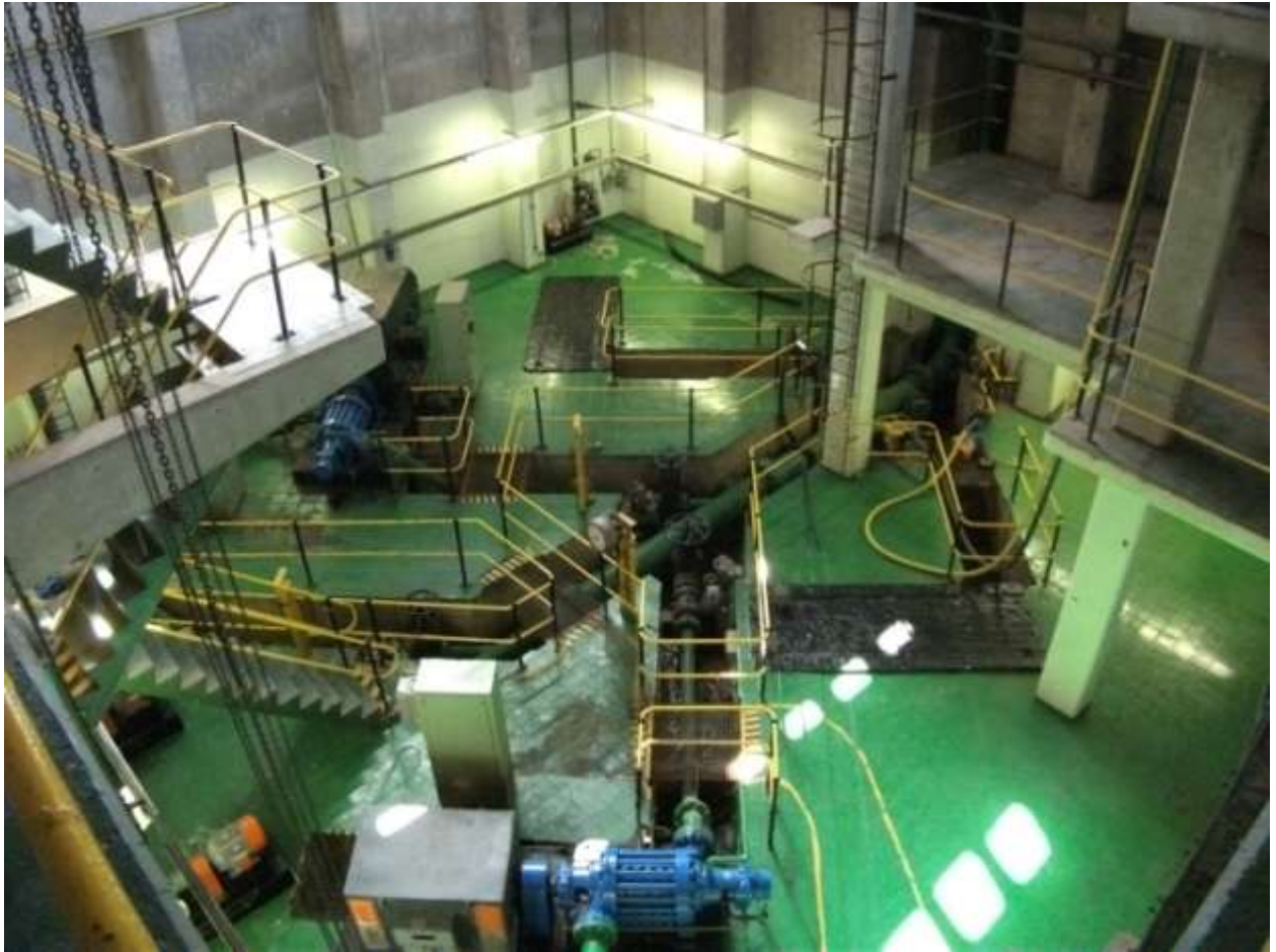
Henkries WTP Potable Water Pump Station
