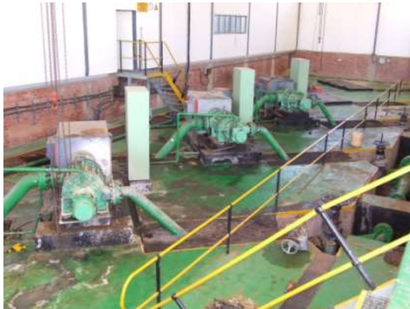
Doornwater In-line Booster Pump Station
