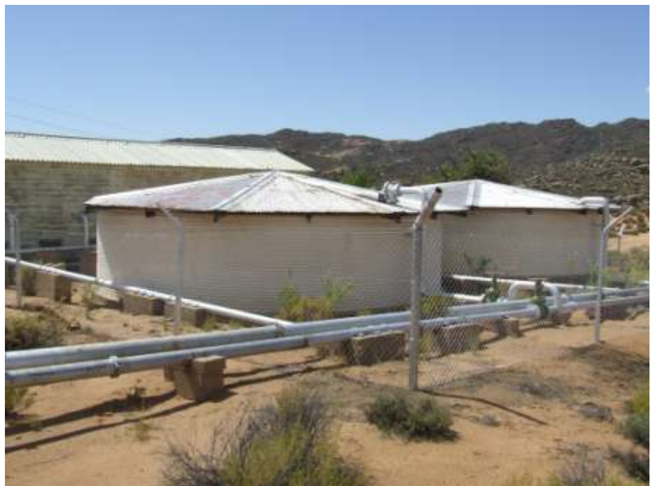
Garagoup Pumpstation and Reservoir Complex
