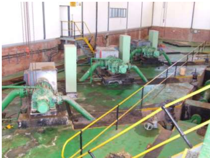
Doornwater In-line Booster Pump Station
