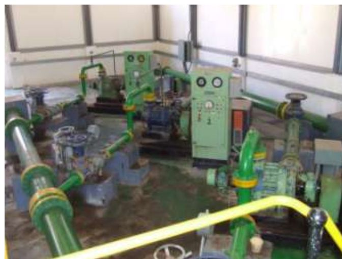
Henkriesmond Booster Pump Station
