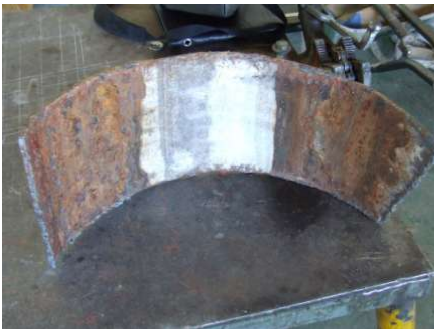
Section cut off from a 520mm diameter steel pipe which recently failed. Corrosion inside the pipe is severe with no evidence of any concrete lining remaining. Wall thickness of the pipe is less than 2mm in the vicinity of the longitudinal weld.
