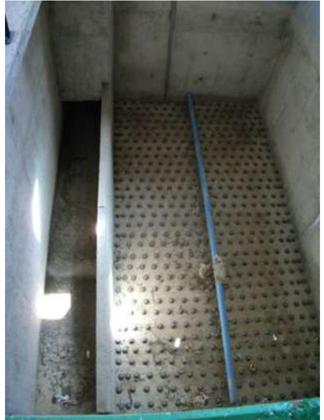
Unfitted spare filter at Henkries WTP
