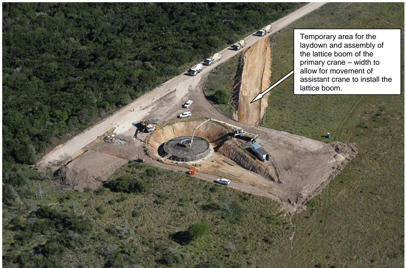
Photo 15 : Aerial view of typical turbine platform, showing the temporary space required for the assembly and dismantling of the long lattice boom of the Primary crane
