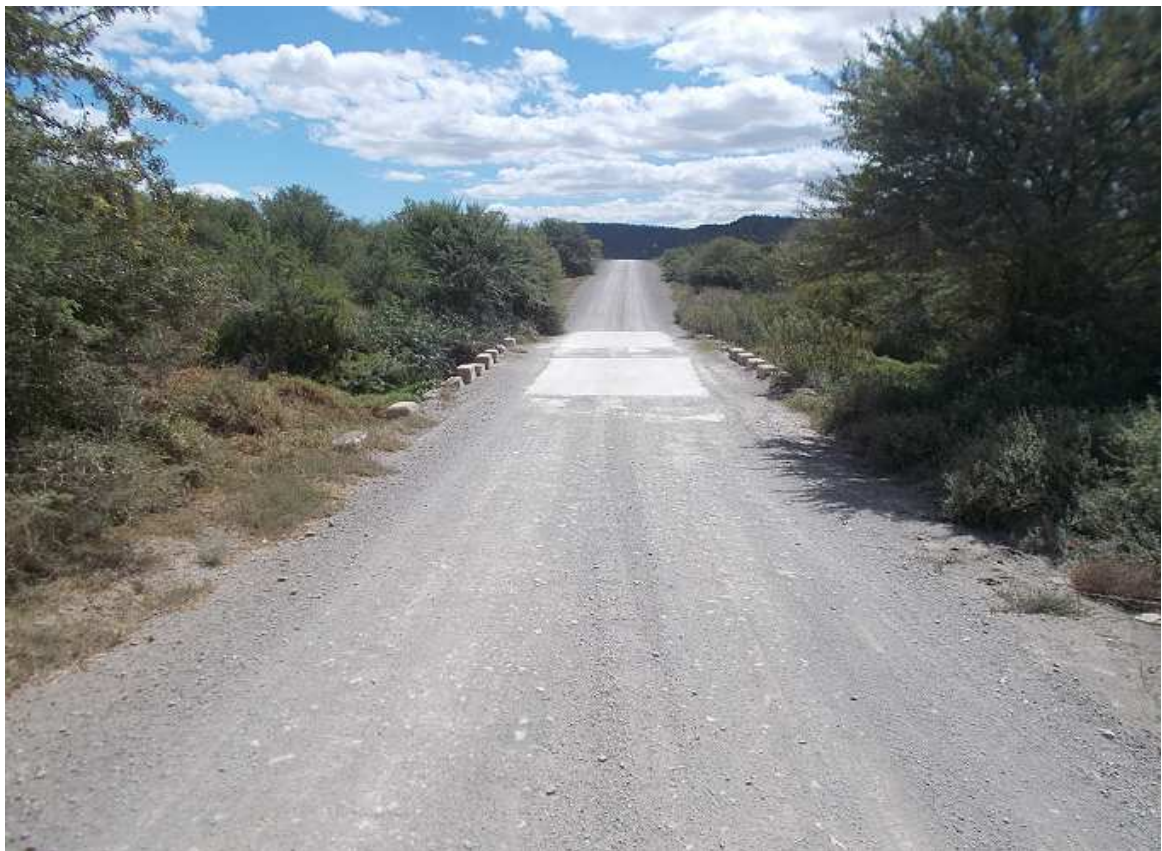
Photo 22: A number of low-level concrete culvert crossings are located along this route. There are noticeable changes in vertical gradients at two of these crossings, which will need to be surveyed and assessed during the Detail Design stage. These sections may need re-alignment, but no upgrading of the culvert structures are required.
