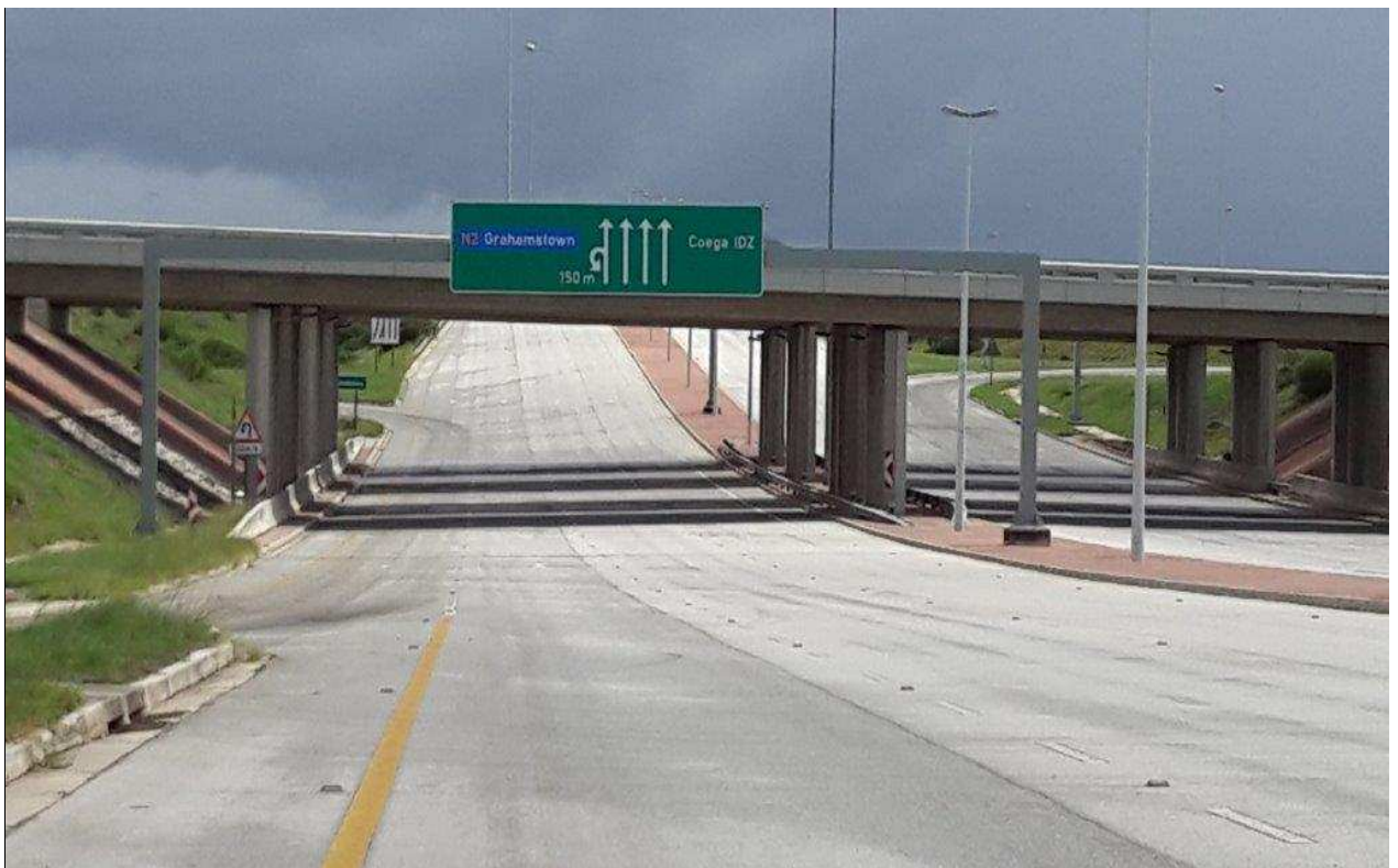
Photo 3: Northern view of the three-lane one-way Neptune road crossing the N2 Bridge. Bridge soffit clearance in excess of 6m is available.
