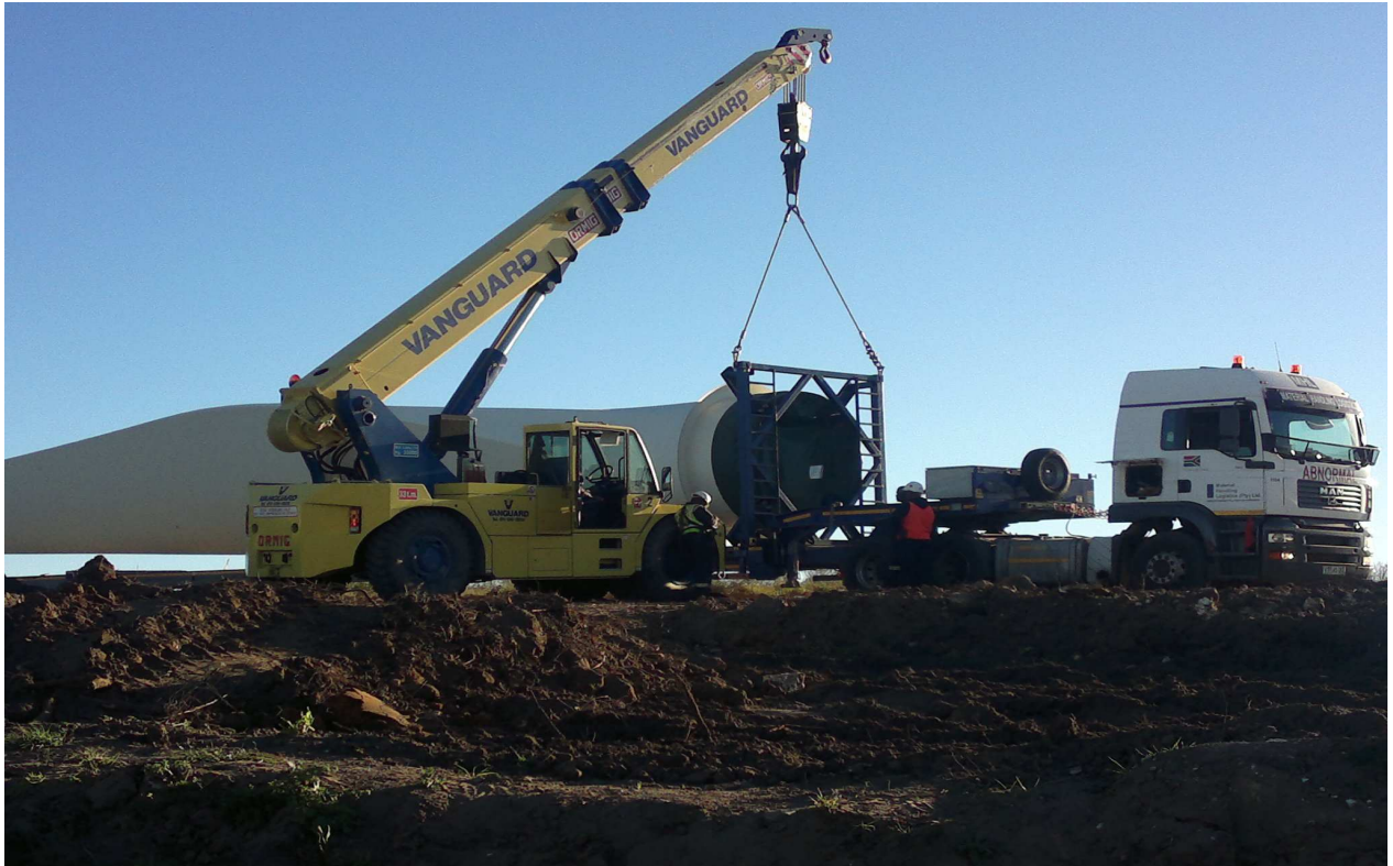
Photo 11 : Small mobile cranes will be required at the turbine off-loading sites, assisting with the safe handling of turbine components.
