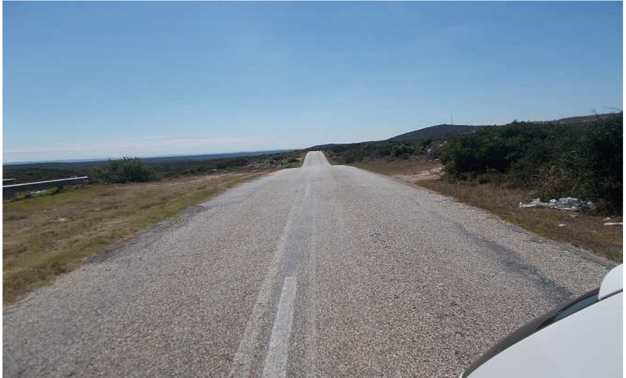
Photo 12: Noticeable crest and sagging vertical curves are present on the Daniel Pienaar Road (R334) between the R367 and R335 intersections. These sections will need to be surveyed to confirm at Detail Design stage that this will not pose transport problems.
