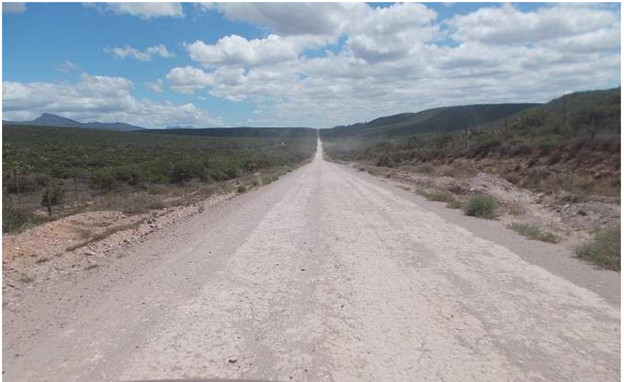
Photo 20: The gravel road (at the time of the assessment) was in a reasonable condition. Upgrading of the road to accommodate transport vehicles will not be required, however regular maintenance(wet grading) will be required during the construction stage.
