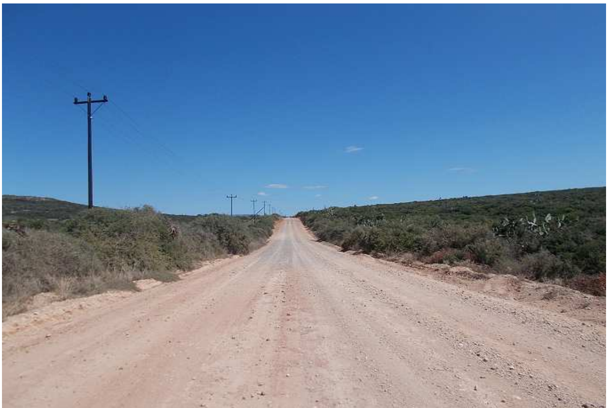
Photo 15: Typical section of the gravel road DR1938 that at the time of the assessment was in a good riding condition. The road is average 5 to 6m wide with some areas exceeding 7m.
