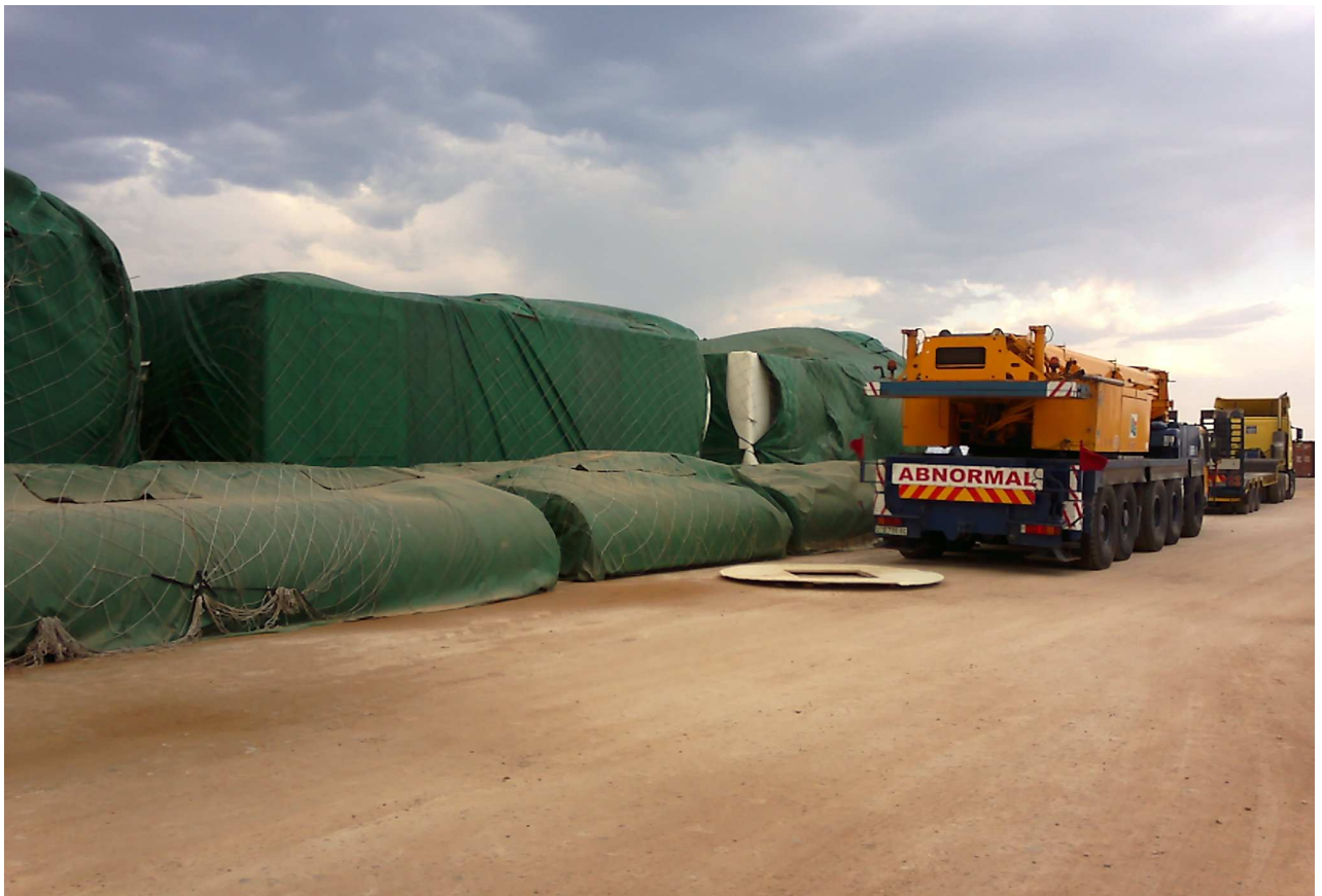
Photo 10 : Mobile cranes parked at a typical centralised wind turbine component laydown storage site.
