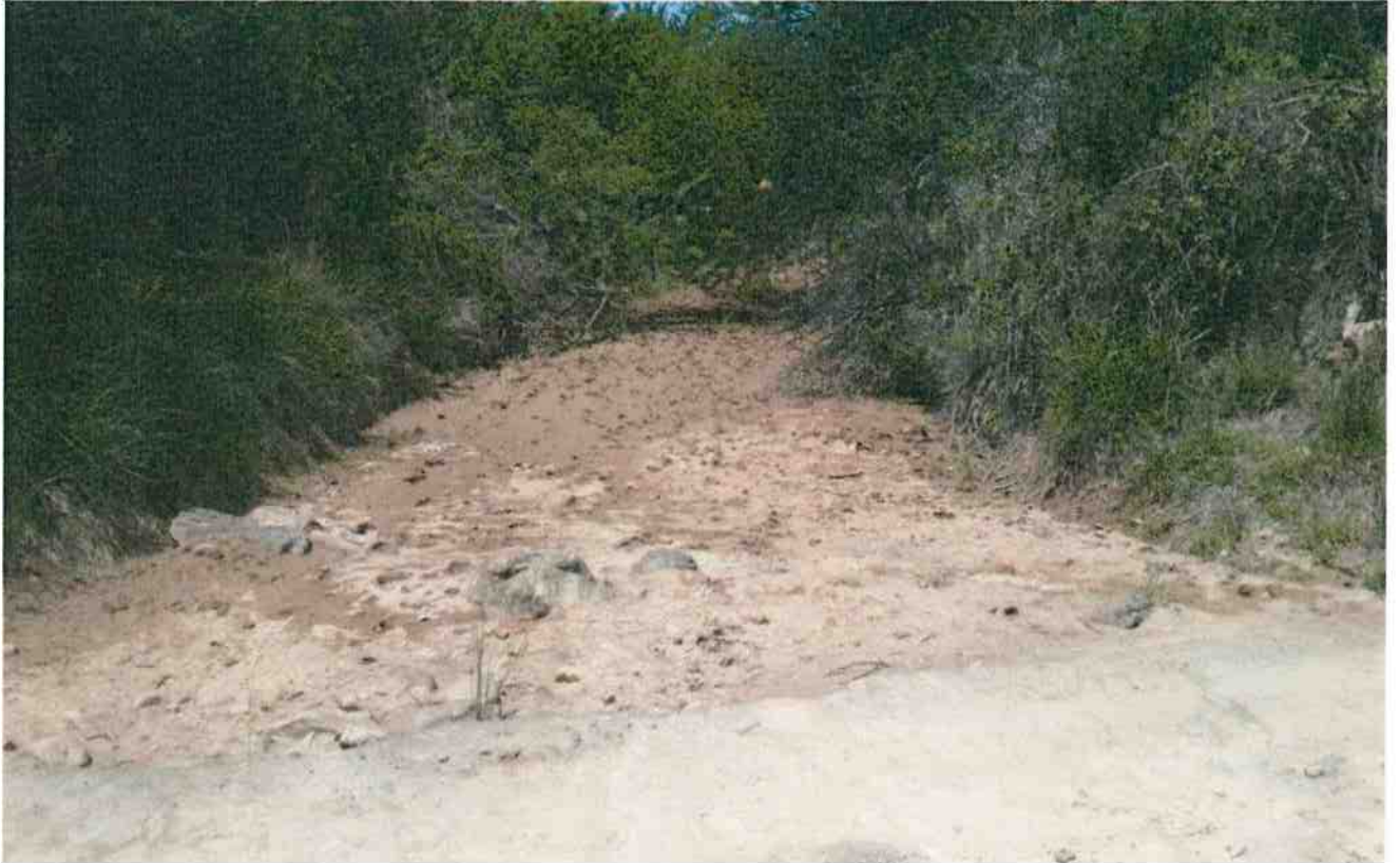
Photo 1 : Typical View of Stream Crossing (non-perennial / dry water course) on the Provincial Minor Road MN 50474. Note sandy river bed and concrete drift in front.
