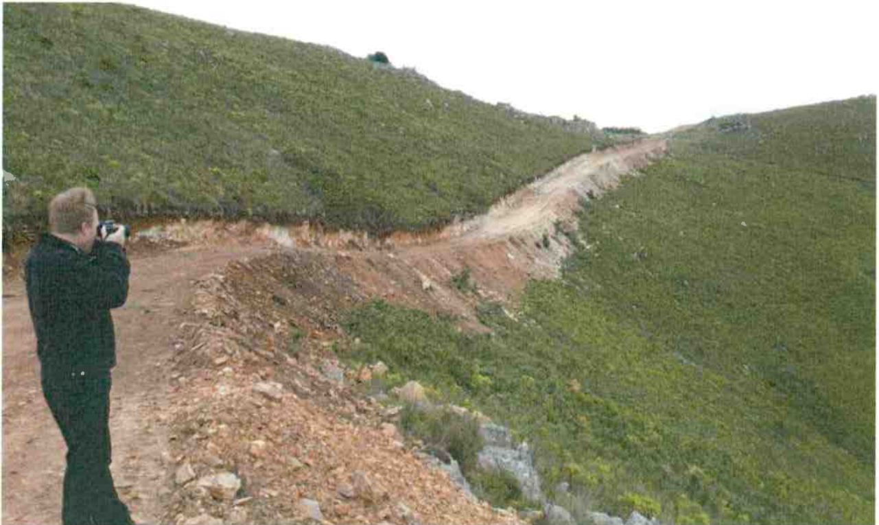
Photo 7 : View of existing gravel road (Provincial Minor Road MN 50475) providing access to the wind farm. Note the fill embankment on lower side of road profile, showing high exposure / risk for erosion damage.
