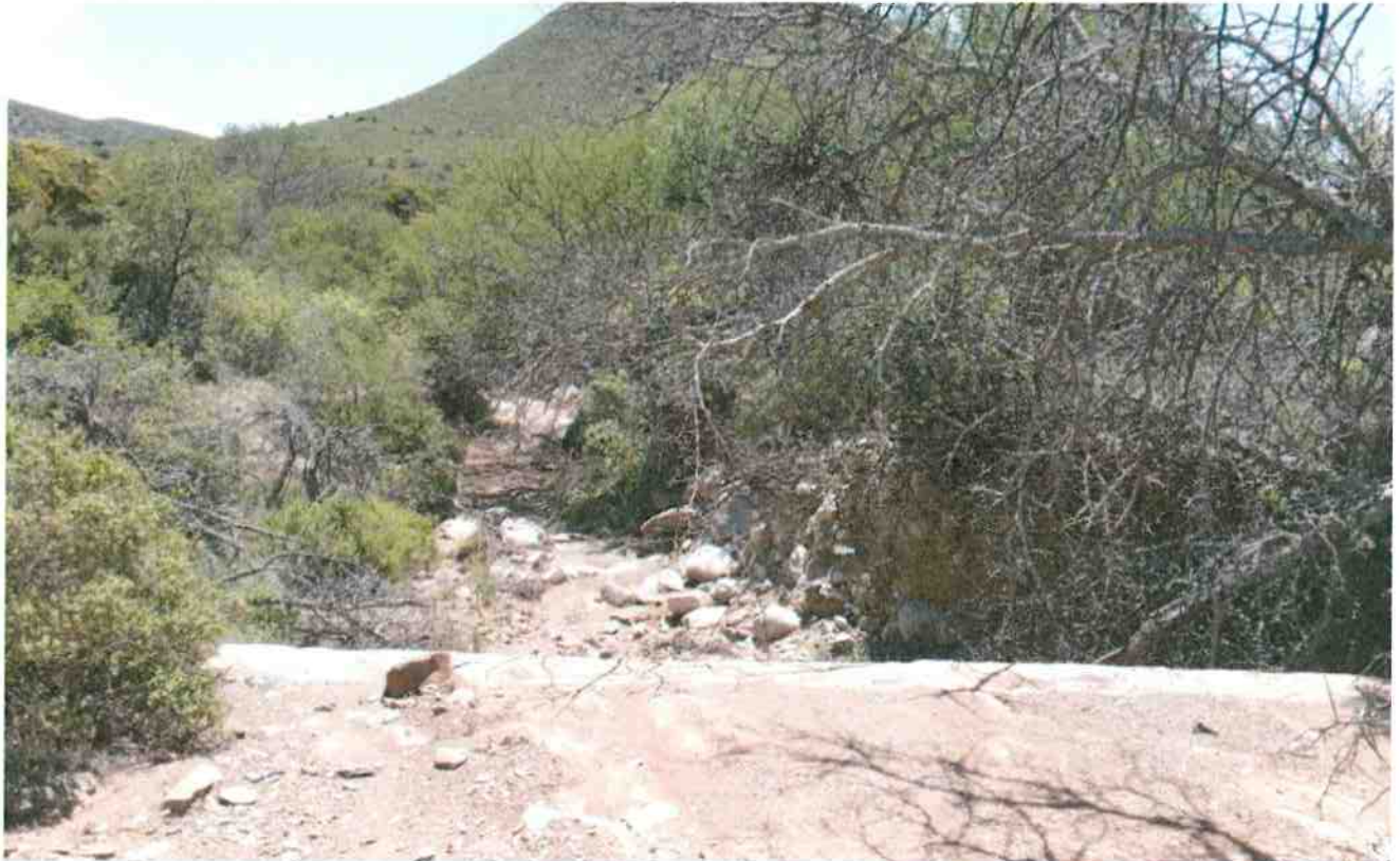
Photo 3 : Typical View of Stream Crossing (non-perennial / dry water course) on the Provincial Minor Road MN 50474. Note sandy river bed with large boulders and concrete drift in front.
