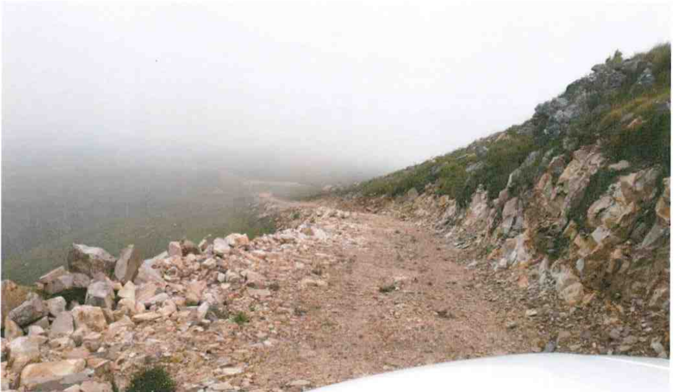
Photo 6 : View of existing gravel road (Provincial Minor Road MN 50475) providing access to the wind farm.
