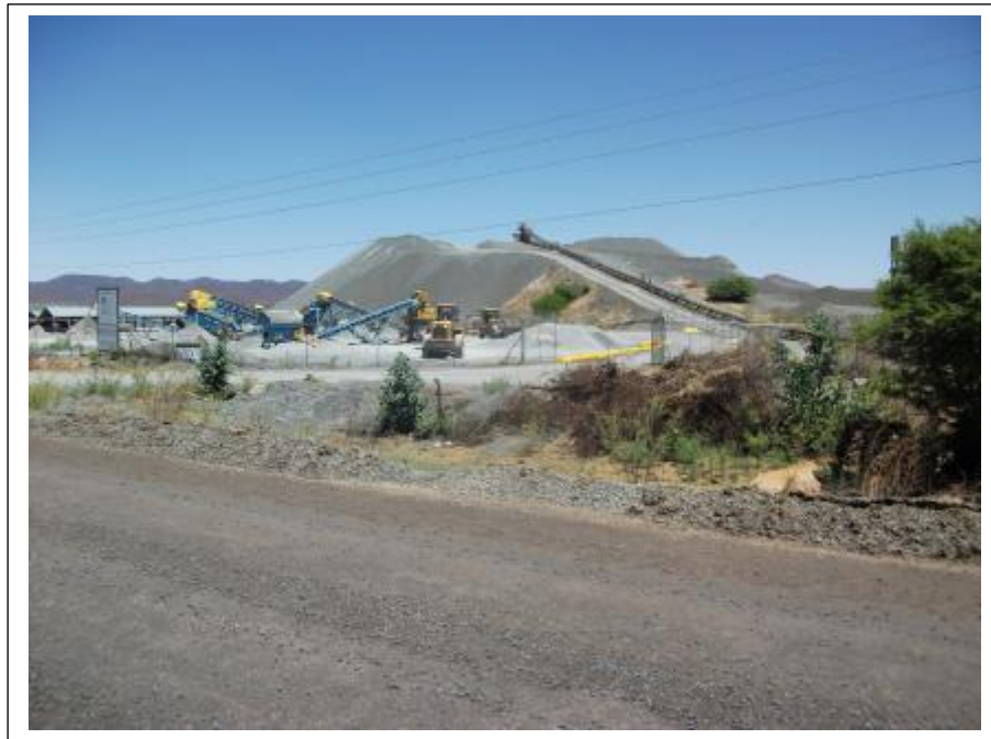
Figure 5- The existing aggregate crusher and part of its footprint. This area was surveyed during earlier heritage studies and no heritage resources were found on this level piece of turf veld (above).
