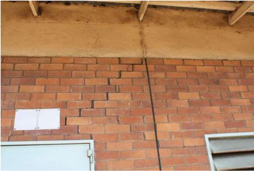
Figure 7: Example of blast induced damage.
