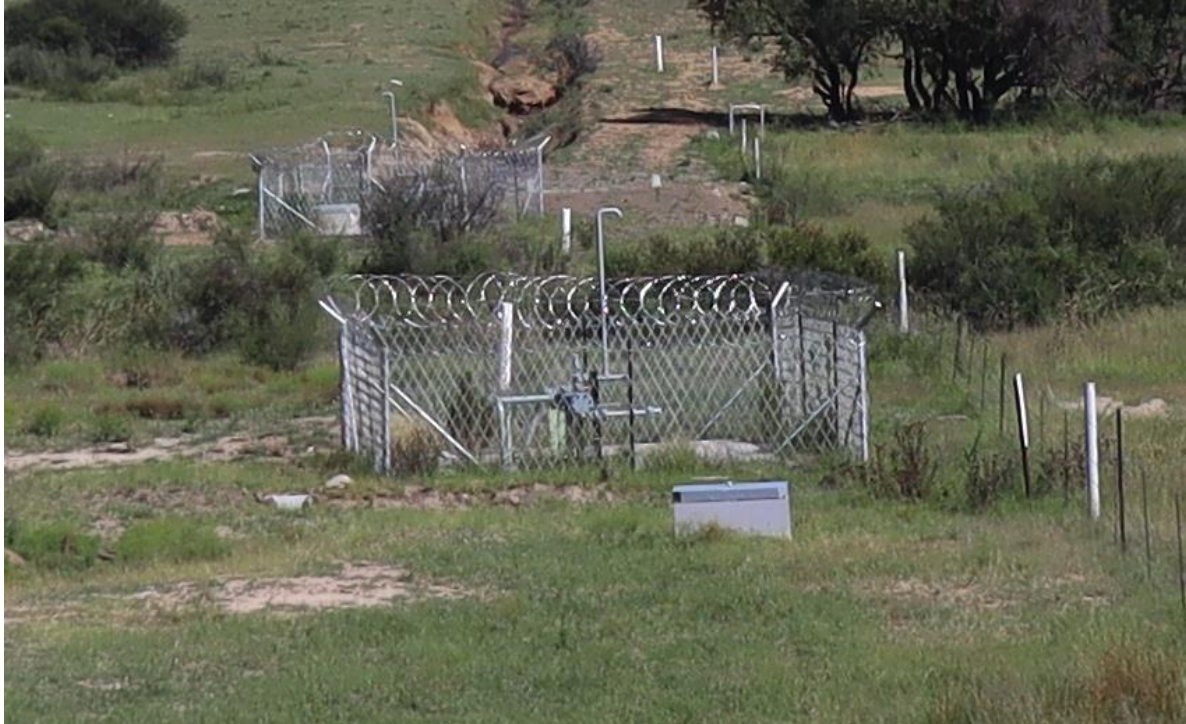
PLATE 19, PHASE 1 OPERATIONAL PIGGING STATION
