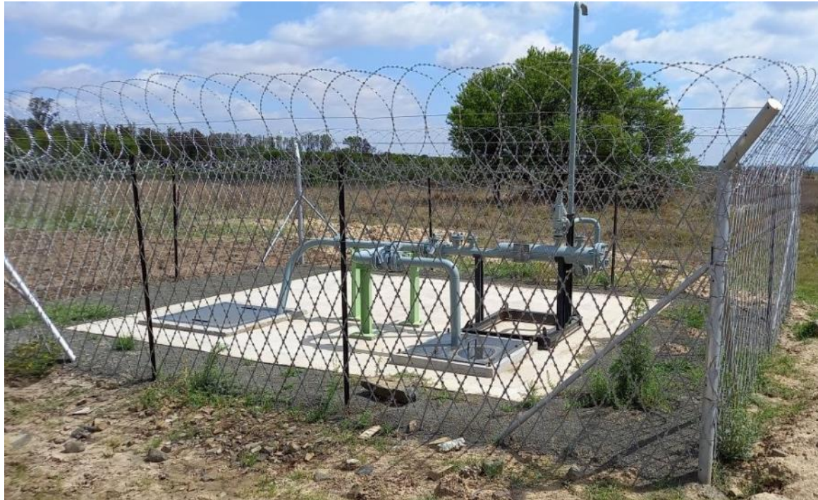
PLATE 5 – VIEW OF EXISTING CLUSTER 1 PIGGING STATION
