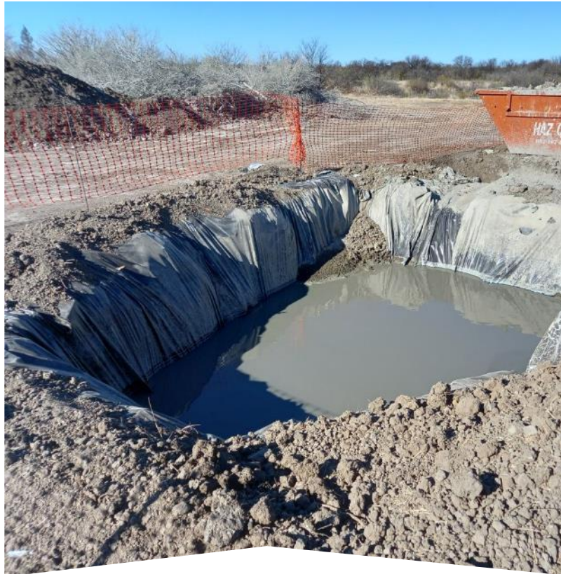
PLATE 1 – TYPICAL AREA OF DISTURBANCE FOLLOWING DRILLING OF EXPLORATION BOREHOLE
