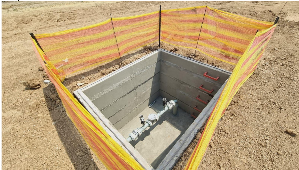
PLATE 2 – TYPICAL CLUSTER 2 WELL INSTALLATION
