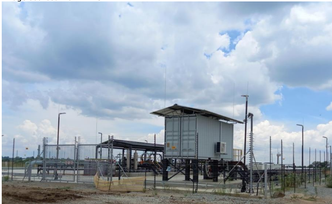
PLATE 6 – VIEW OF EXISTING CLUSTER 1 COMPRESSOR STATION
