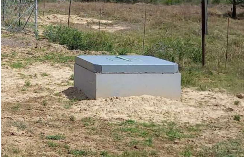
Figure 10: View of an existing low point drain constructed as part of Cluster 1.
