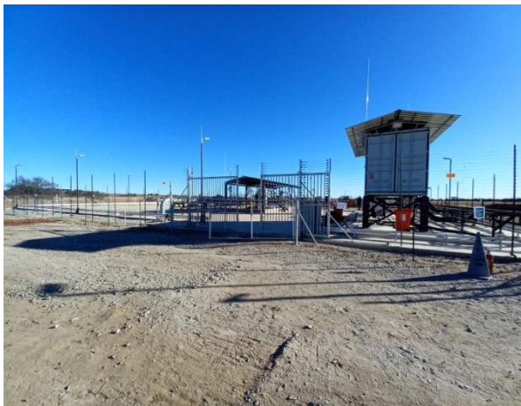
Figure 11: Centralised Compressor station.
