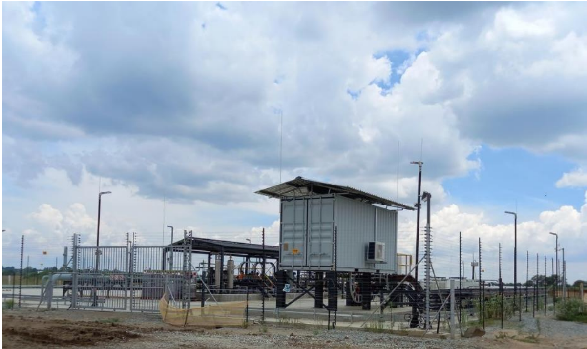
Figure 7: Example of Compressor Station constructed as part of Cluster 1.
