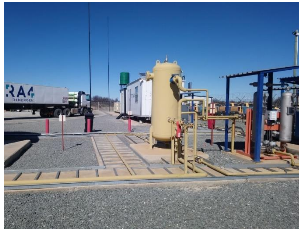
Figure 18: HDR1 Production well and associated facility.
