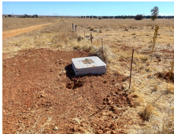
Figure 12: Low point drain.
