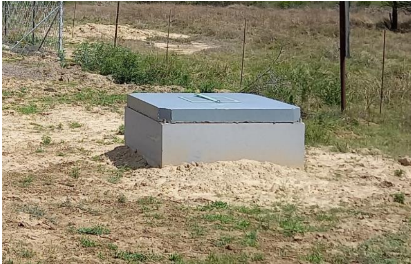
Figure 5: View of an existing low point drain constructed as part of Cluster 1.
