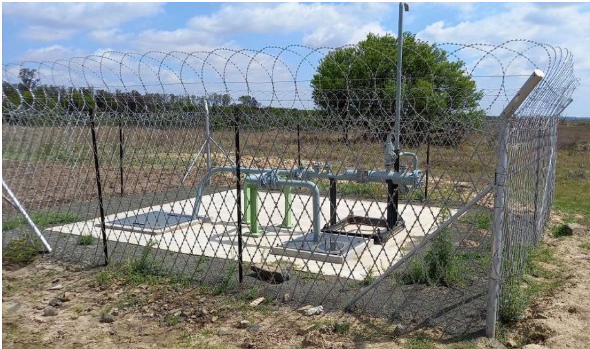
Figure 4: View of an existing pigging station constructed as part of Cluster 1.
