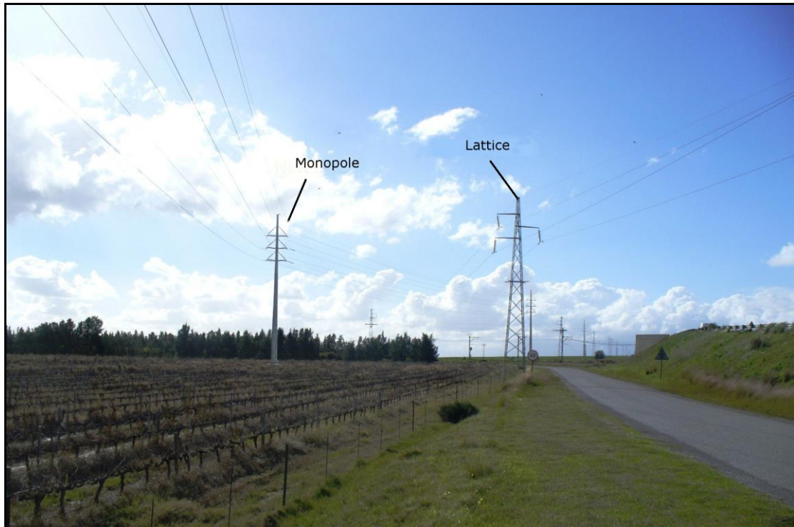
Figure 3: Longer distance view of power line towers.
