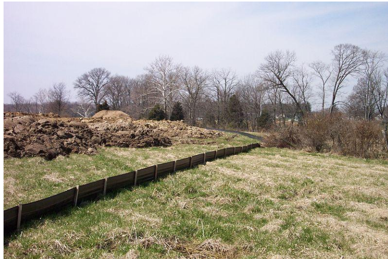
Figure 25: A siltation screen below a construction site to prevent the movement of sediment downstream (image from www.wikipedia.com )
