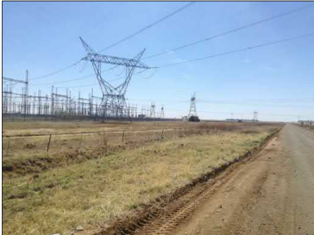
Figure 17: High voltage power lines feeding into Perseus Substation.
