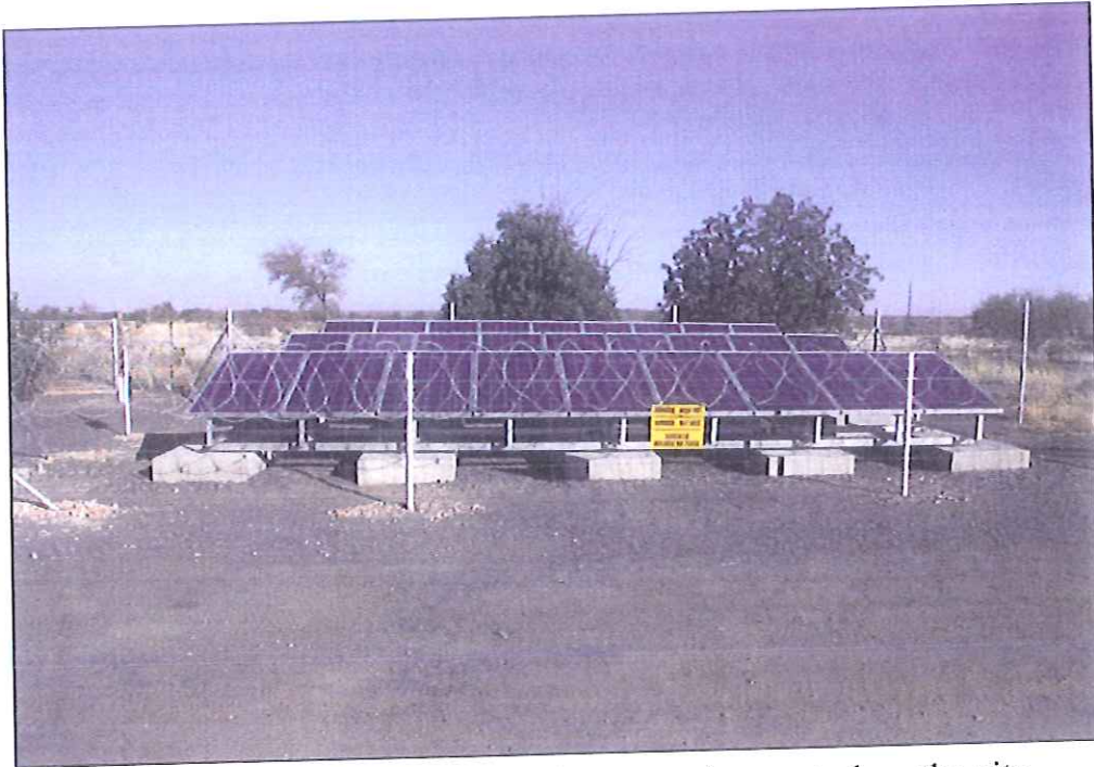
Pilot PV solar plant similar to the one to be erected on the site.
