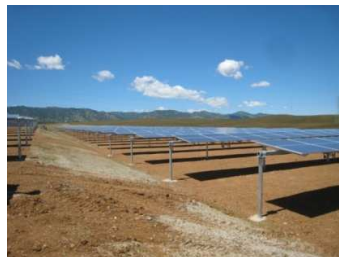
Fig 2.3. Image of Ray tracker utility scale solar tracker installation., tech option 1. Source Mulilo
