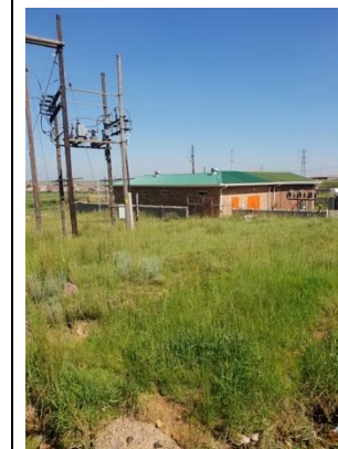
Substation. (26°00'16.2" S 29°02'23.0"E)
