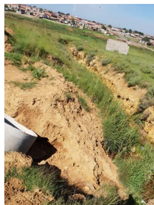
Soil erosion. (26°00'16.3"S; 29°02'19.4"E)
