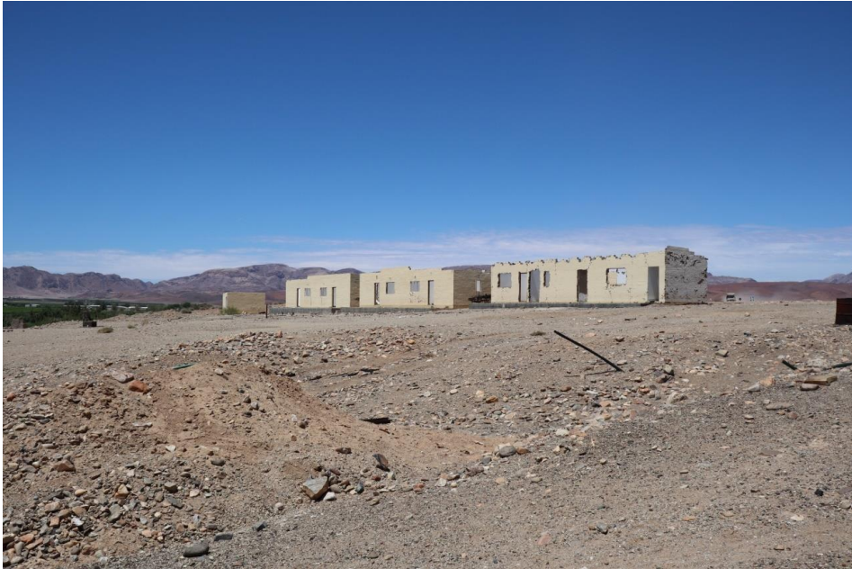
Plate 18, Existing accommodation block buildings that will be repaired and reused during the mining phase
