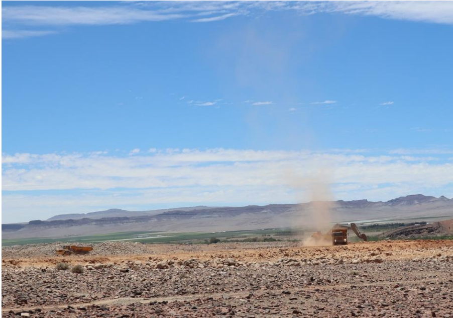
Plate 25, Excavation plant is likely to be made more obvious by dust
