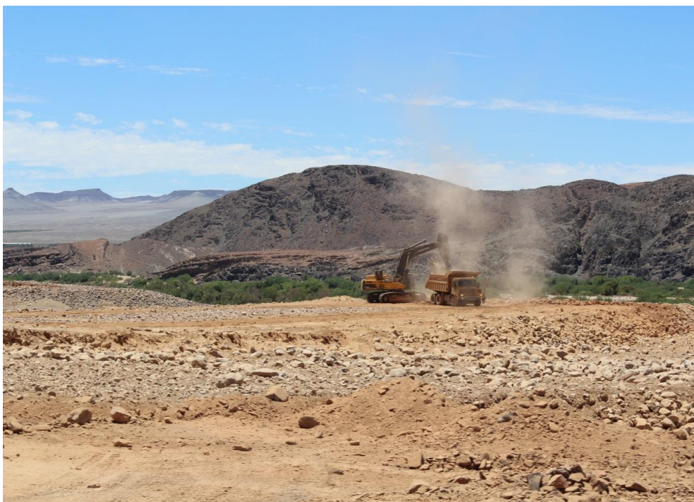
Plate 5: Excavator and dump truck used to extract gravels to load and haul to static processing plant
