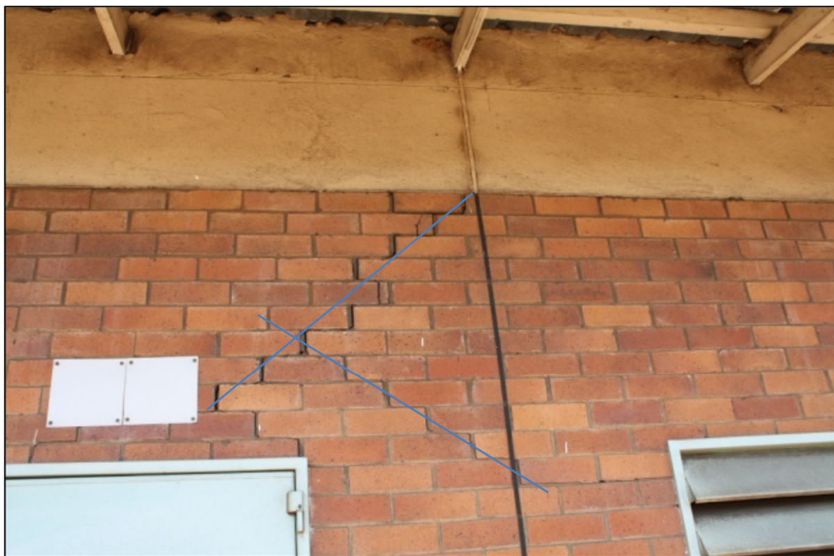
Figure 6: Example of blast induced damage.
