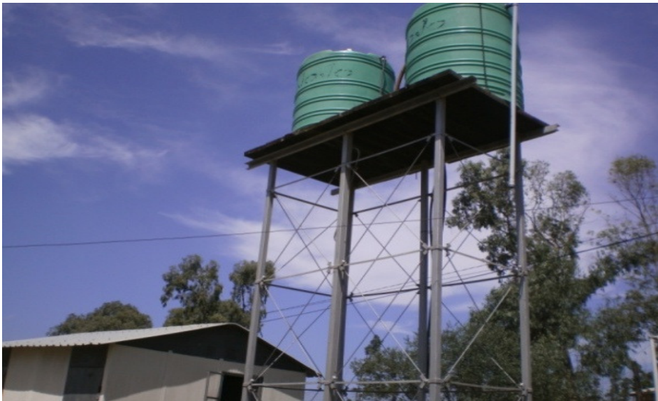
Fig. 11 Water tanks adjacent to Crime Prevention Office
