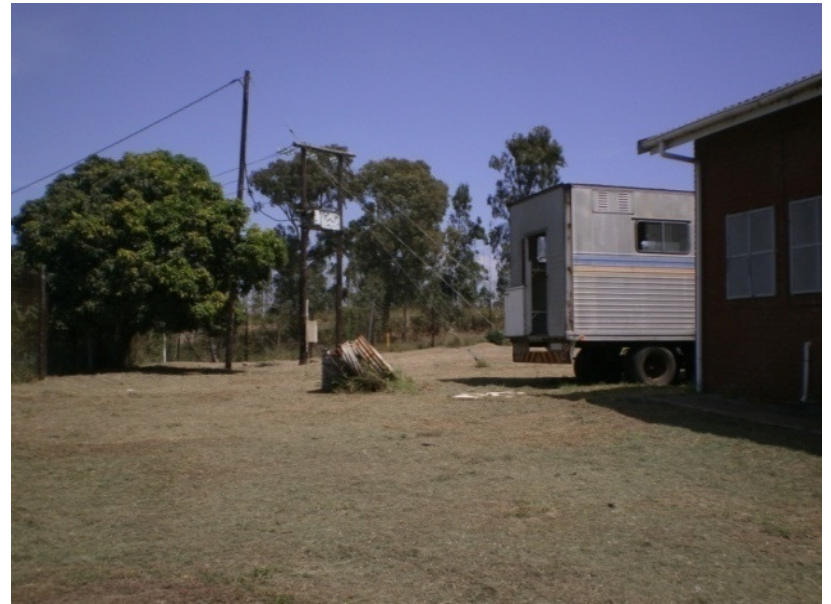
Fig. 12 Electricity power lines within the site
