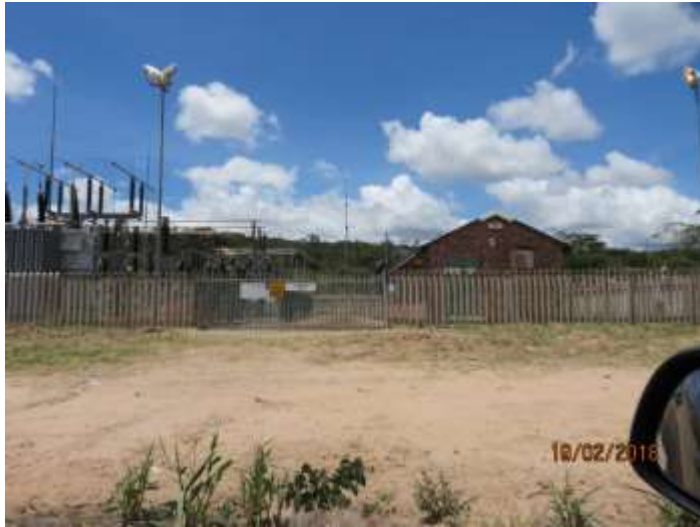
Photo 1: The existing Matsafeni Substation from where the project will start and the new powerline will be constructed.
