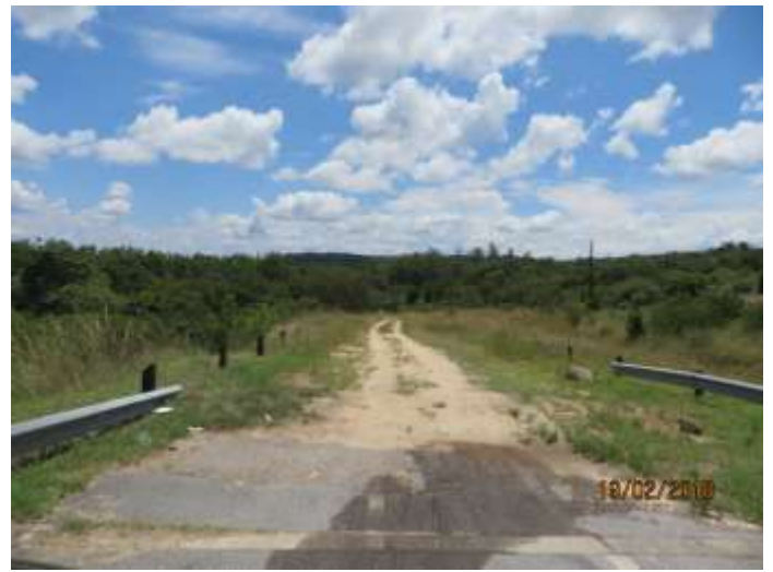
Photo 16: Access road to Croc Substation. The road will be paved to allow for heavy vehicle transport to and from the substation.
