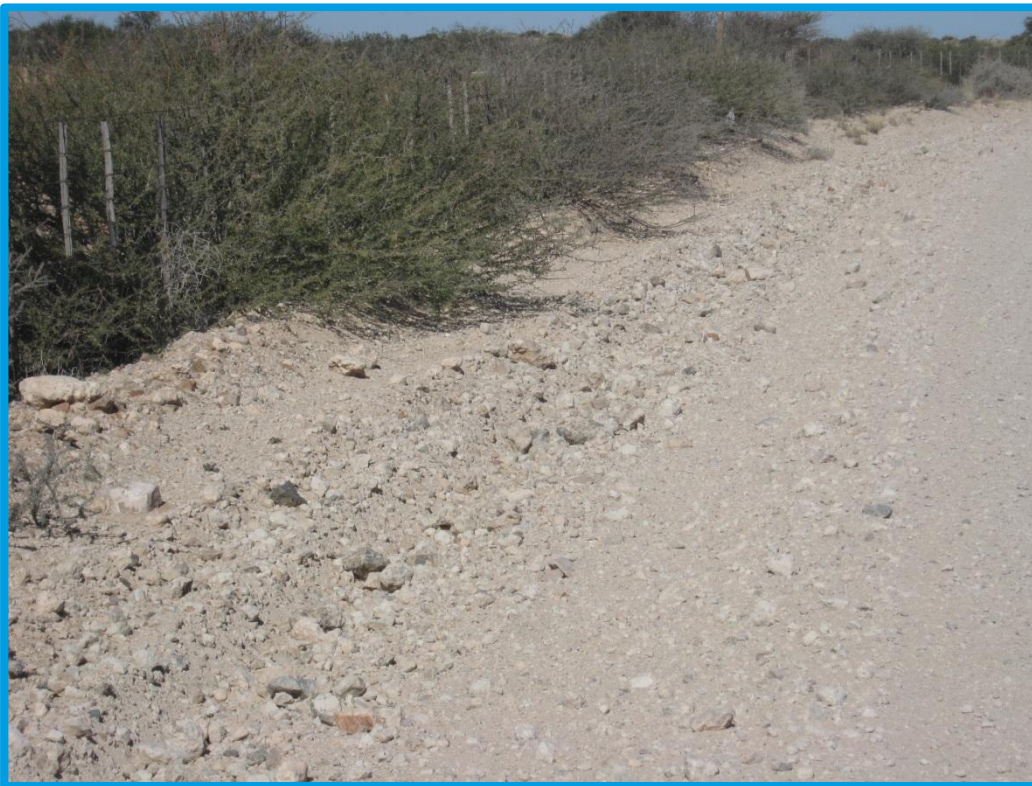
Photograph 16: Loose material on the DR3322 provincial road
