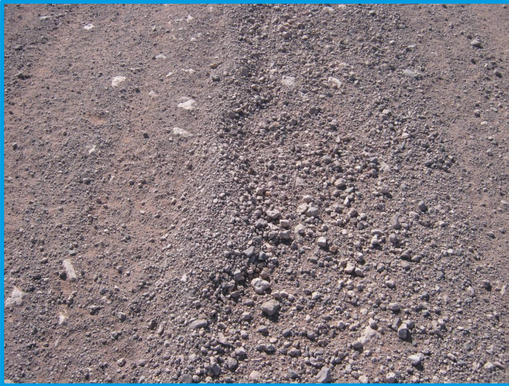
Photograph 15: Loose material on the DR3322 provincial road
