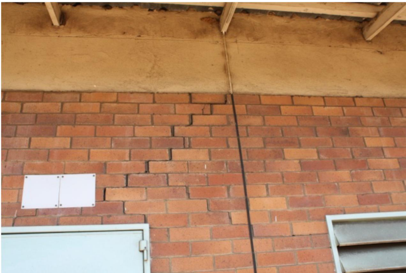
Figure 8: Example of blast induced damage.
