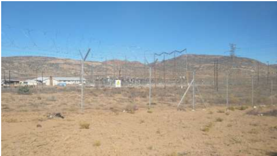
FIGURE 22 NAMA SUBSTATION OUTSIDE OF SPRINGBOK
