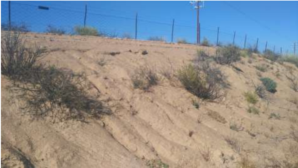
FIGURE 36 EROSION NEXT TO ROAD, IN NAMAQUALAND KLIPKOPPE SHRUBLAND
