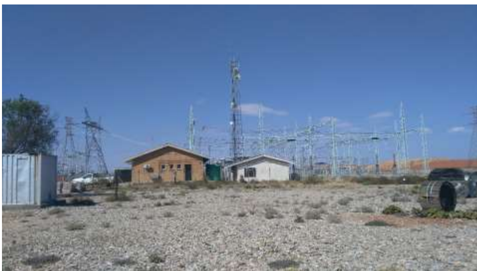
FIGURE 43 VIEW OF A PORTION OF THE GROMIS SUBSTATION
