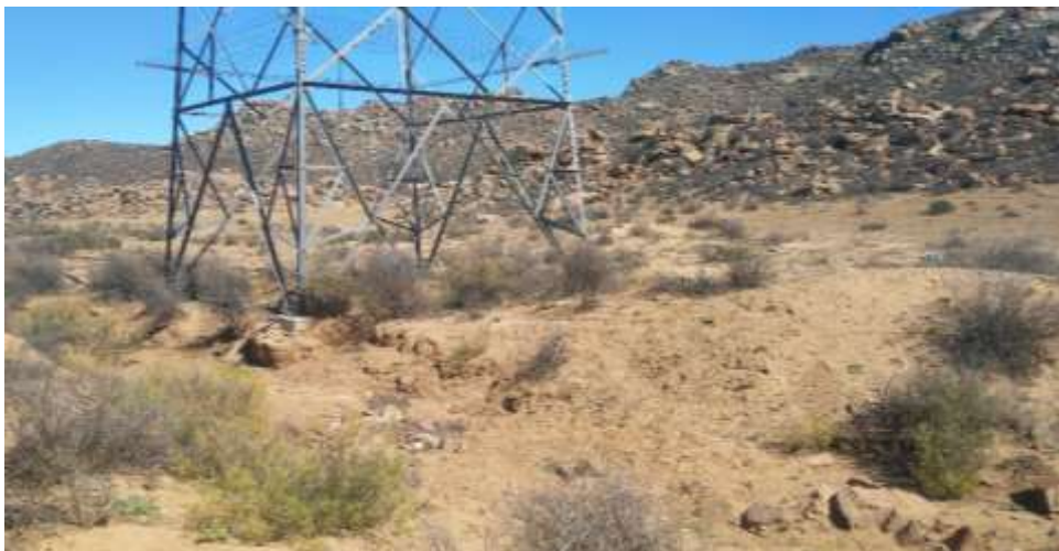
FIGURE 25 EROSION AROUND THE BASE OF AN EXISTING PYLON
