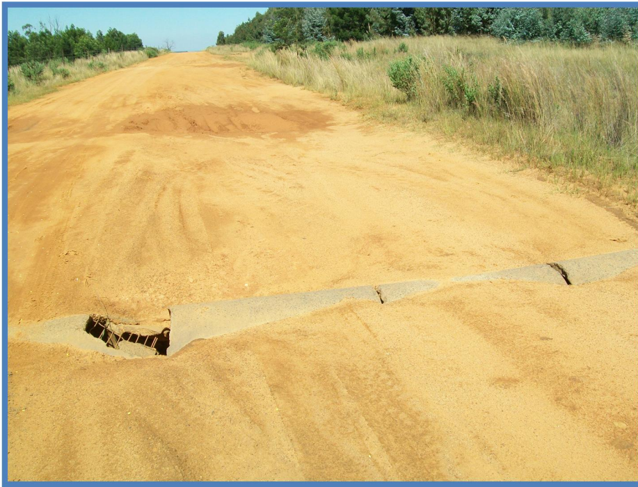
Photo 10: Damaged drainage pipe
