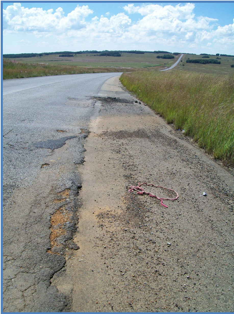
Photo 7: Paved Shoulder with Shoving of Asphalt and Base Failure
