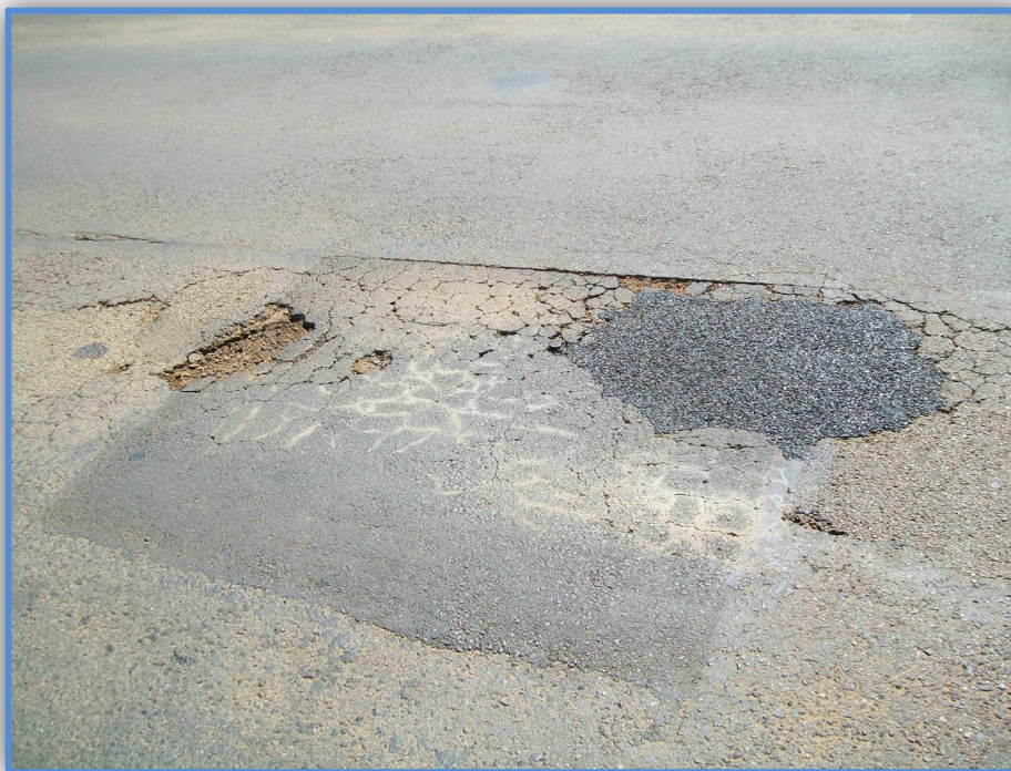
Photo 4: Surface Cracks and Pumping that lead to Potholes
