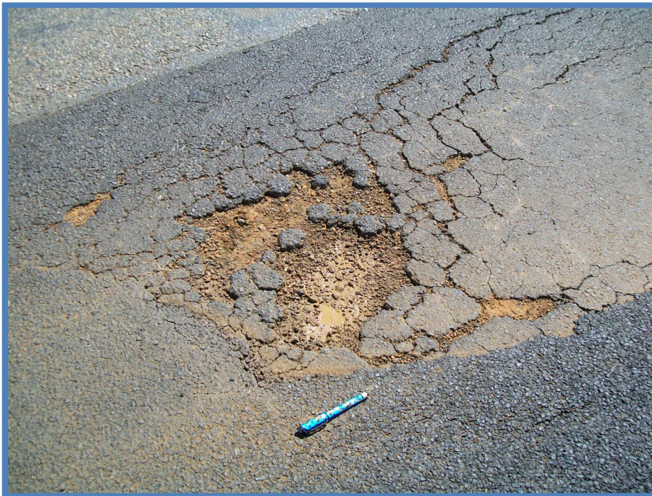
Photo 6: Water Retained in Pothole after Rain
