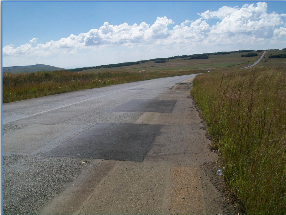
Photo 3: Severe Patching Along the R555 East of the Site
