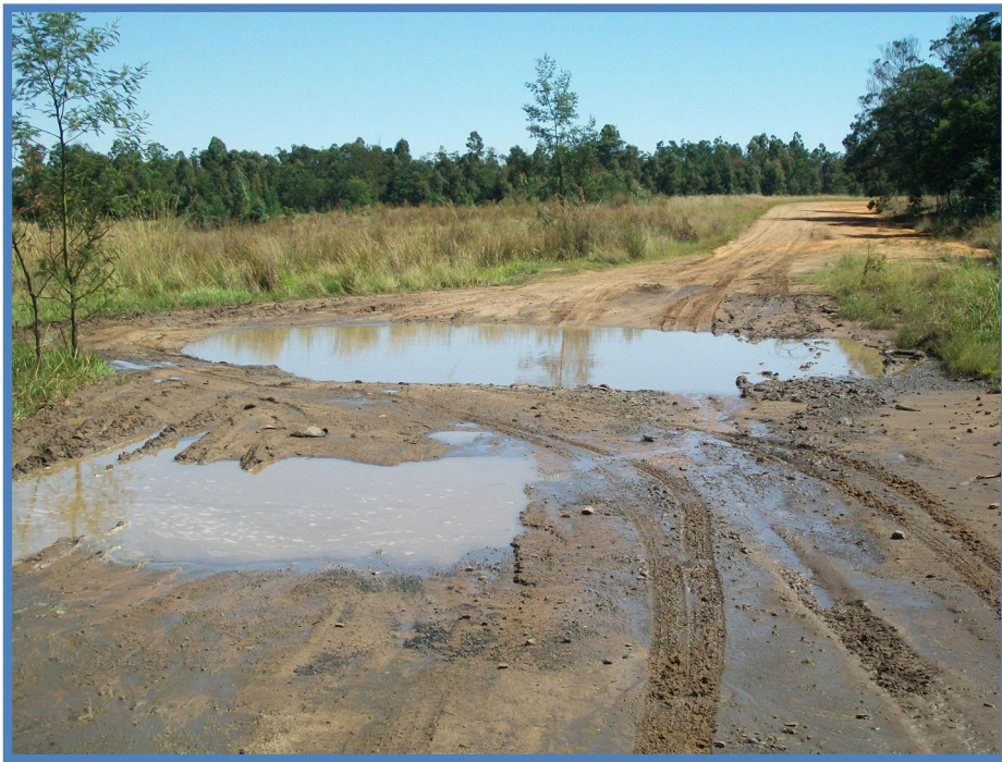
Photo 9: Pooling water after rain on the D1433_080
