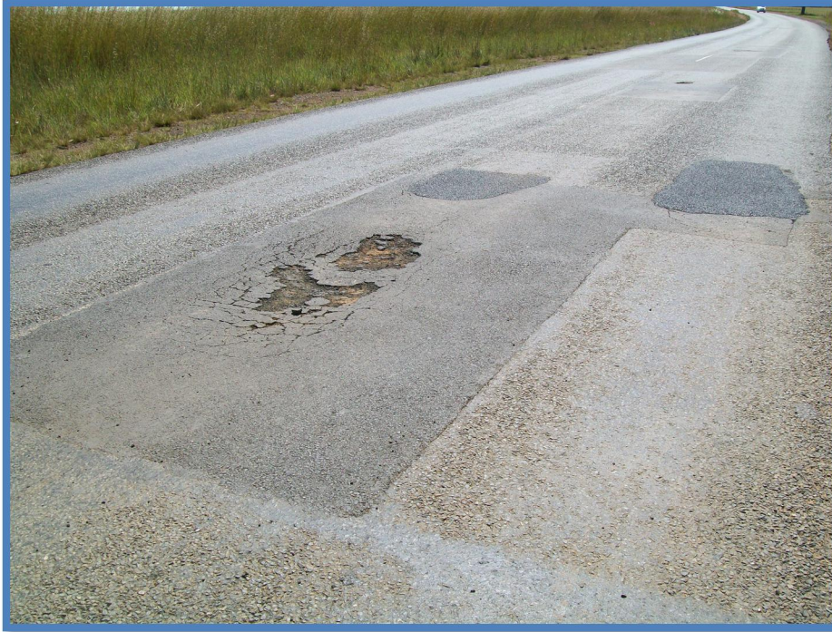
Photo 5: Failure Leading to Potholes in Existing Patching
