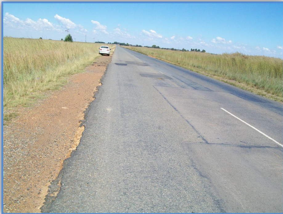
Photo 2: Edge Breaks along Gravel Shoulder
