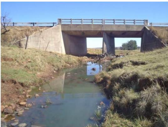
Downstream view of the Selons River site RV2 near the R555 bridge (October 2011).
