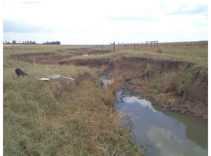
Figure 5: Downstream view of the Selons River site RV1 indicating bank side erosion (October 2011).
