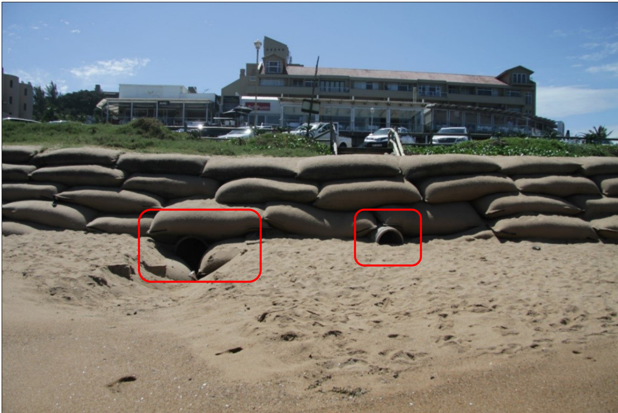
Plate 1. The existing stormwater outlets that get blocked.
