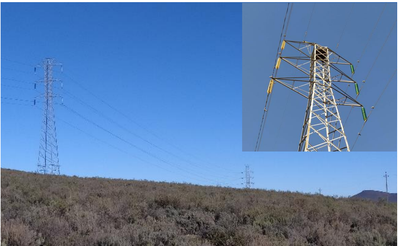
Figure 6: A high voltage line running through the northern part of the PAOI, with a Martial Eagle nest (insert)
