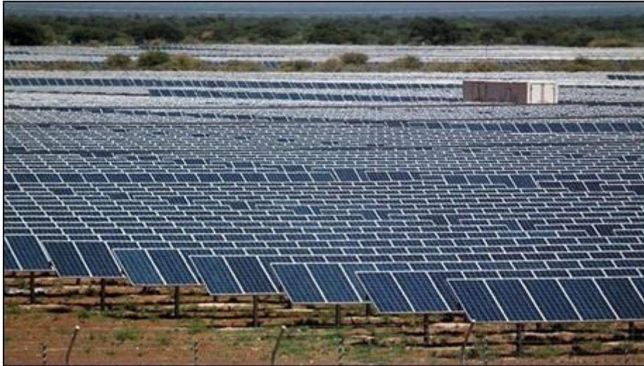
Figure 20: Kathu Solar Power Plant (photo courtesy of “visits to the park”), near Kathu, Northern Cape Province.
