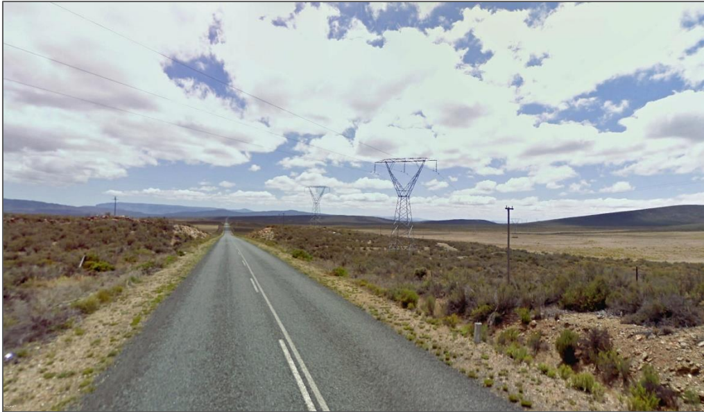
Figure 19: 132kV powerlines traversing the norther sector of the study area as seen from the R318 main road (Source: Google Earth 2022).
