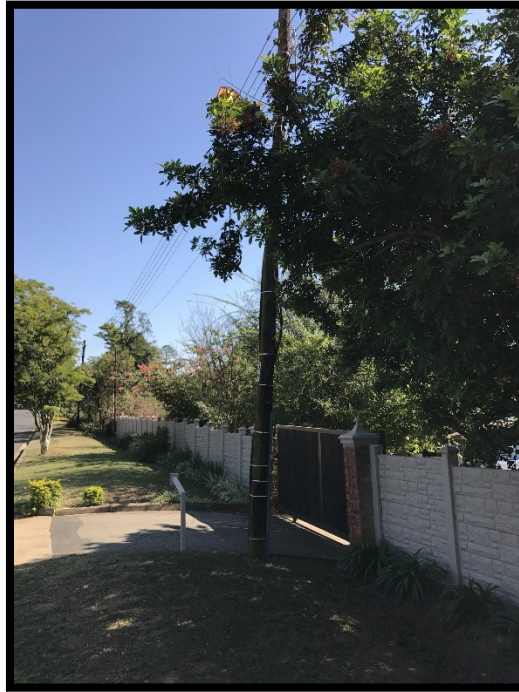
This photo shows the existing overhead electrical cable situated along Grimthorpe Avenue
