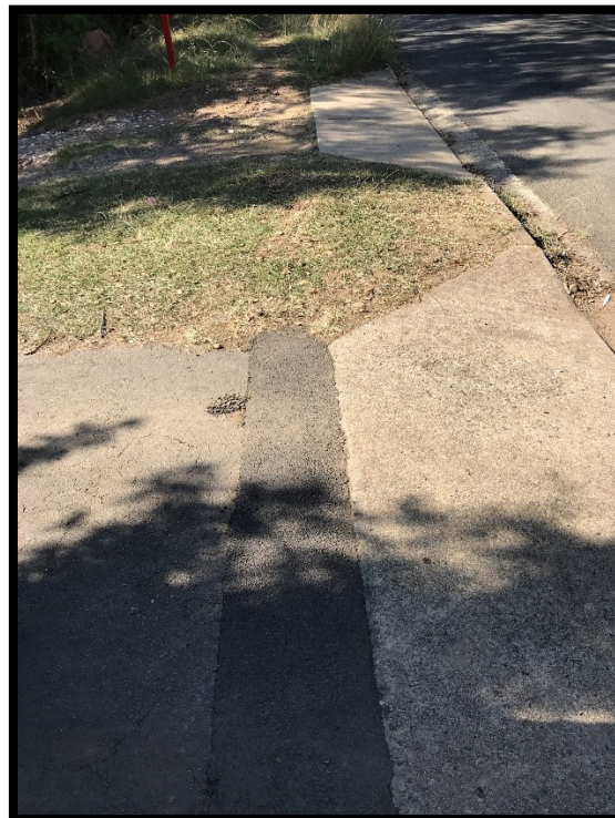
This photo shows the newly laid asphalt where the 225mm Ø distribution main was laid
