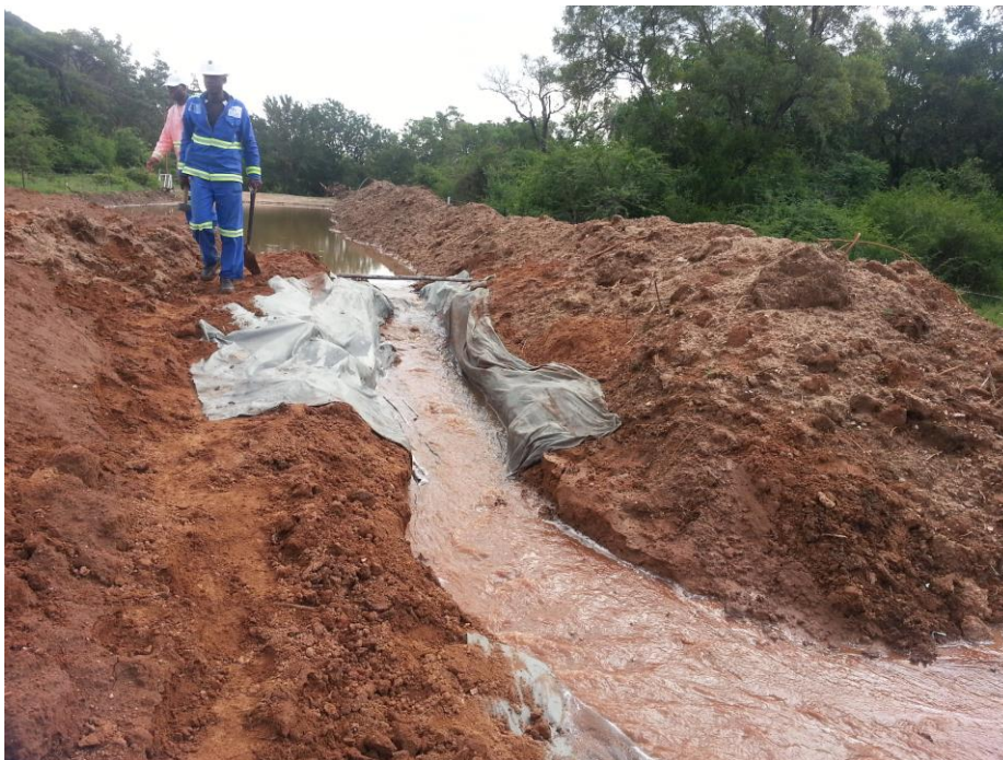
Photo 2. Lining of soil stockpiles prior to release of pooled storm water to ensure no loss of stockpile.
