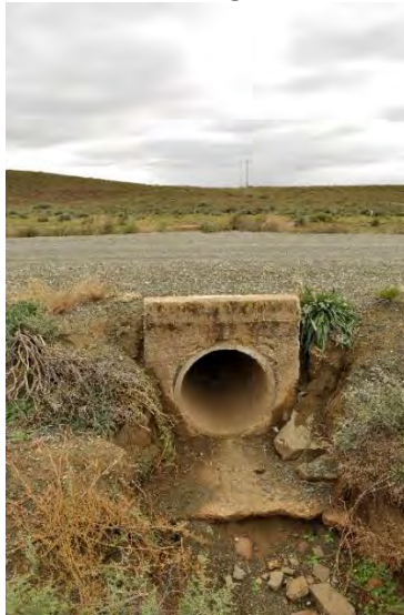
Plate 2: A view of an existing pipe culvert crossing on the R356 (32.7817023S 20.3044875E)
